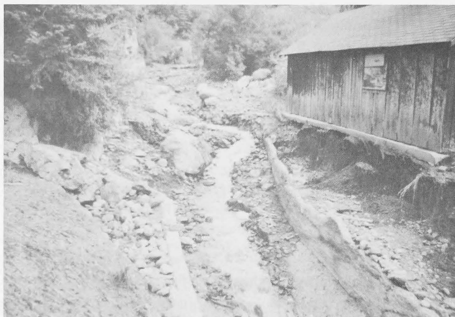
Figure 34. Portland Creek flume entrance, 1982. The flume shows damage from past events. The building on the right is spattered with mud from the 1982 event.
