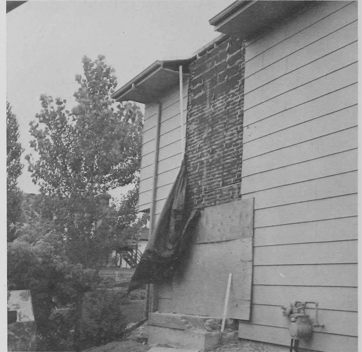
Figure 32. The chimney of this house located in a southwest Denver suburb separated from the house and had to be removed before it collapsed. It was damaged by swelling soils.
