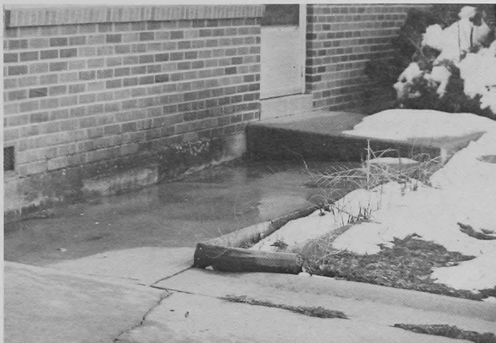
Figure 27. Settlement of the fill material has resulted in reversed drainage next to the foundation.
