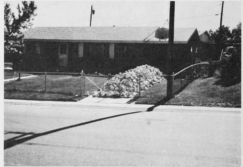
Swelling soils damaged this basement slab so severely that the concrete was removed. The photo shows the basement floor before it was hauled away.
