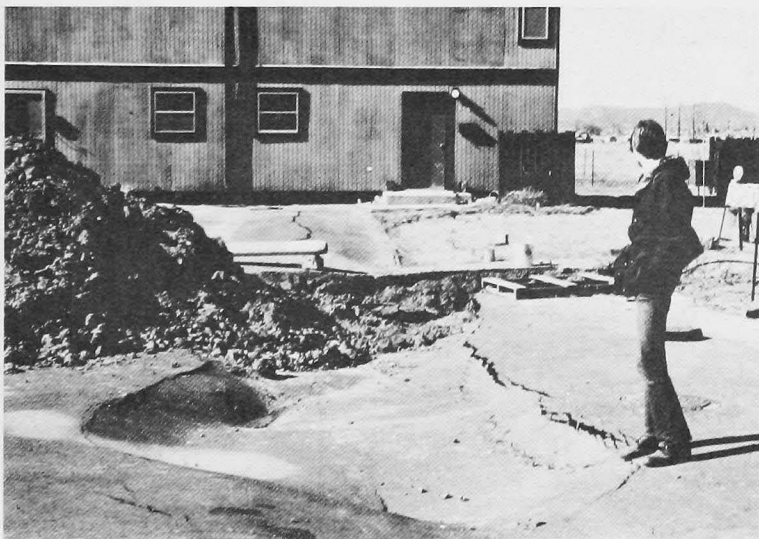
Hydrocompaction of soils caused by a ruptured water line in Boulder County.
