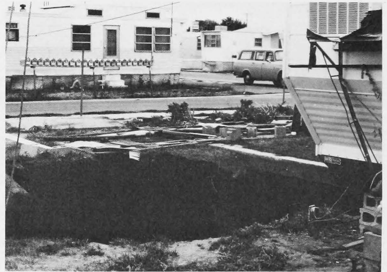
Subsidence pit in a trailer park at Lafayette. This 25 ft x 25 ft hole, 30 ft deep resulted from collapse of the overlying materials into an inclined mine shaft.
