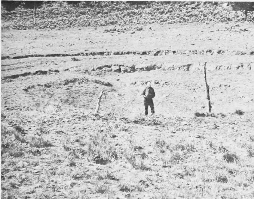
Figure 28. A SURFACE DEPRESSION RESULTING FROM HYDRO-COMPACTION. INITIALLY A SHALLOW EXCAVATION WAS DUG FOR A FARM POND. AFTER THE POND WAS FILLED, THE AREA BEGAN TO SUBSIDE, AND SUBSIDENCE CONTINUED FOR ABOUT TWO WEEKS UNTIL THE POND WAS DRAINED. NOTE THE COMMONPLACE AND APPARENTLY HARMLESS APPEARANCE OF THE COLLUVIAL MATERIAL IN THE FOREGROUND AND AT A DISTANCE BEHIND THE MAN.
