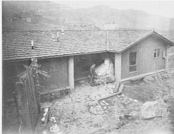
Figure 15. A BLOCK OF ROCK ROLLED DOWNHILL AND DAMAGED THIS HOUSE. WHAT MIGHT HAVE HAPPENED IF THE ROCK HAD BEEN LARGER OR IF IT HAD ROLLED DOWN A STEEPER SLOPE?
