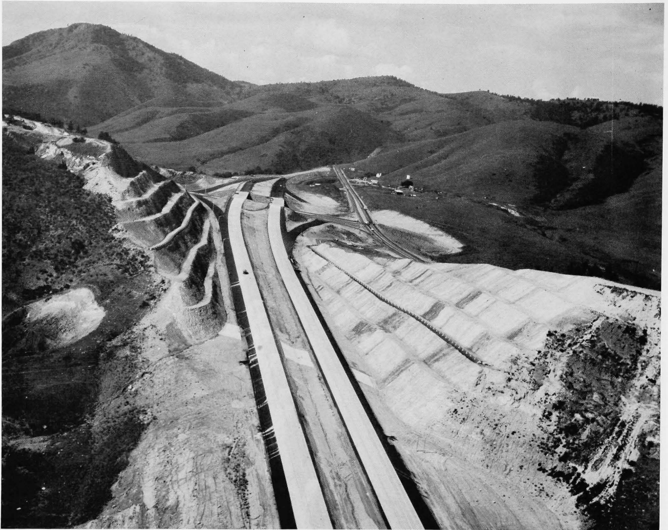
Figure 5. Cut on Interstate Highway in layered sedimentary rocks of the foothills region.
