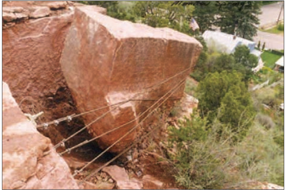
Figure H: A precarious rock above Manitou Springs started to move in 1995 after a period of wet weather. As an emergency measure, high-strength steel cables were wrapped around the rock and anchored to the surrounding ledge to arrest the movement. (Photo by Jon White.)
