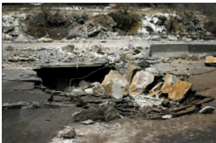
Figure F: Westbound deck of I-70 with extensive damage.
