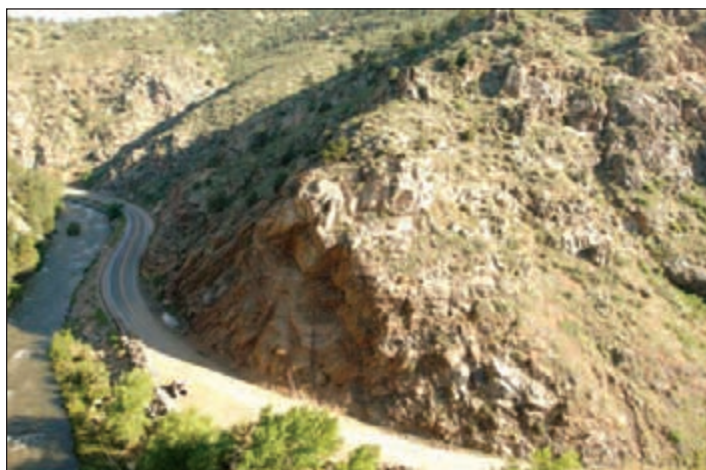
Figure H: Oblique aerial photo of rockslide area after clean-up, before stabilization project. Note the overhanging, unstable rock. (Photo by CDOT.)
