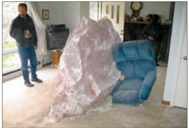
Figure B: In April 2004, this rock from the source area shown above smashed through the wall of a home and came to rest against an easy chair. The homeowner built a rockfall protection fence afterwards. (Photo taken in 2004 by Steve Vanderleest, City of Glenwood Springs.)
