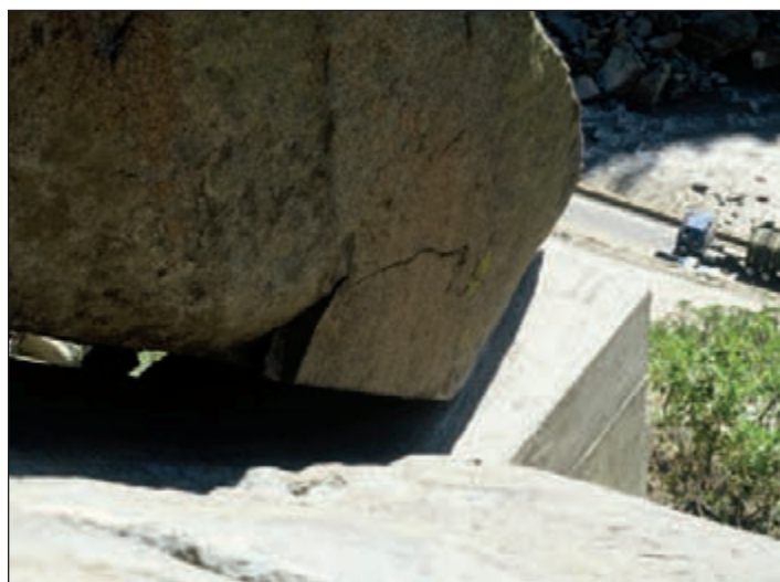
Figure 14: Smaller, upslope concrete buttresses are anchored to the rock face with rockbolts. Then, concrete rebar and wood forms are wired to the anchors in Glenwood Canyon. The concrete is carried in mud buckets by helicopter. The three photos show the progression of the installation. (Photos by Jon White.)
