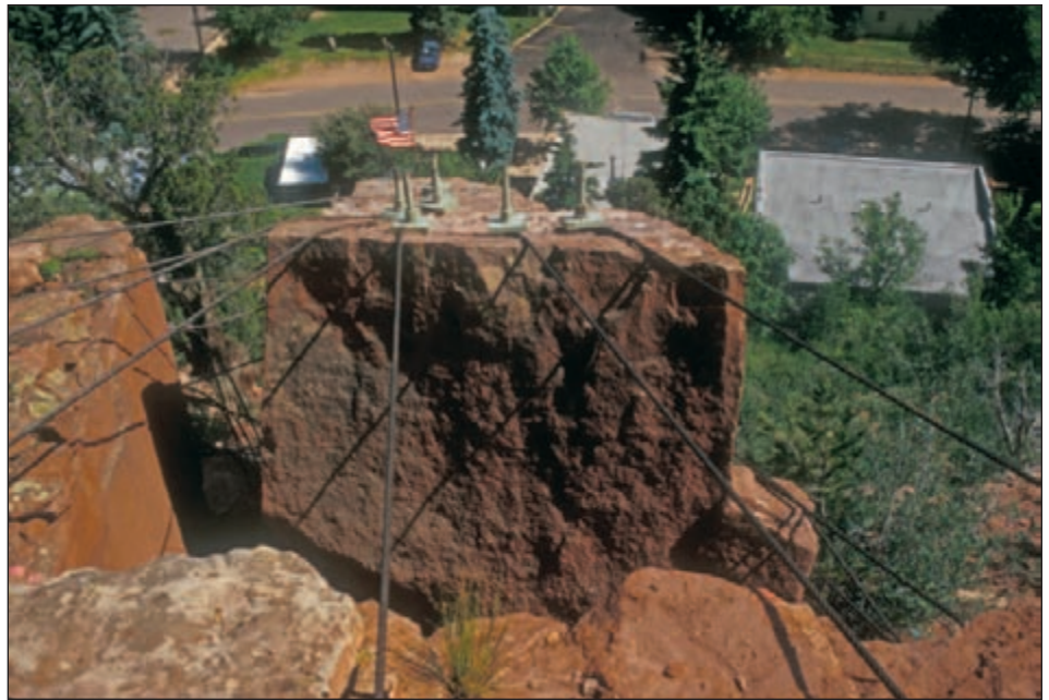
Figure I: After the rock was stabilized, additional cables were physically attached to the top of the rock block and secured to surrounding stable rock. (Photo by Jon White.)
