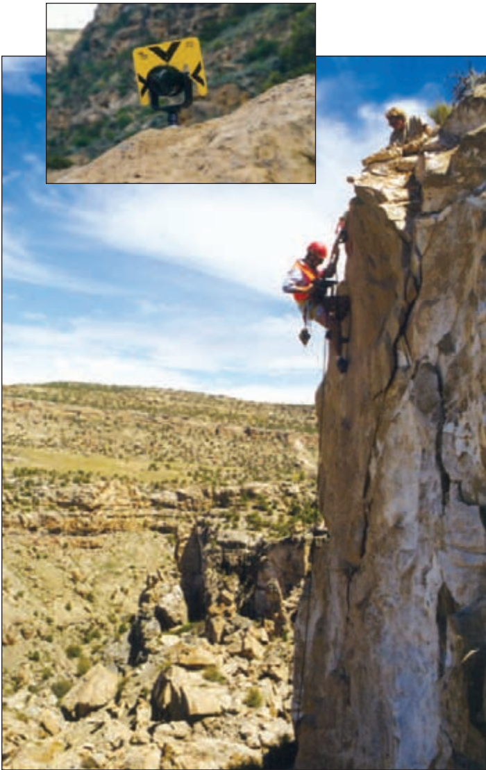
Figure 9: Installation of target prism anchored to a cliff to measure rock movement. Prism is screwed into a wedge anchor bolt that is installed into a drill hole. (Photos by Jon White.)
