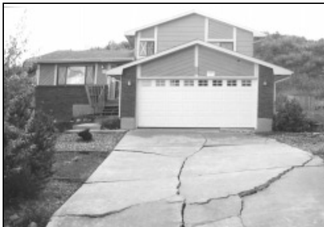
The Colorado Springs area has numerous places with landslide-prone ground and ancient and modern landslides. One of these is in the Holland Park neighborhood in the north-central part of the City. Several homes were damaged or destroyed in this area this past summer.
