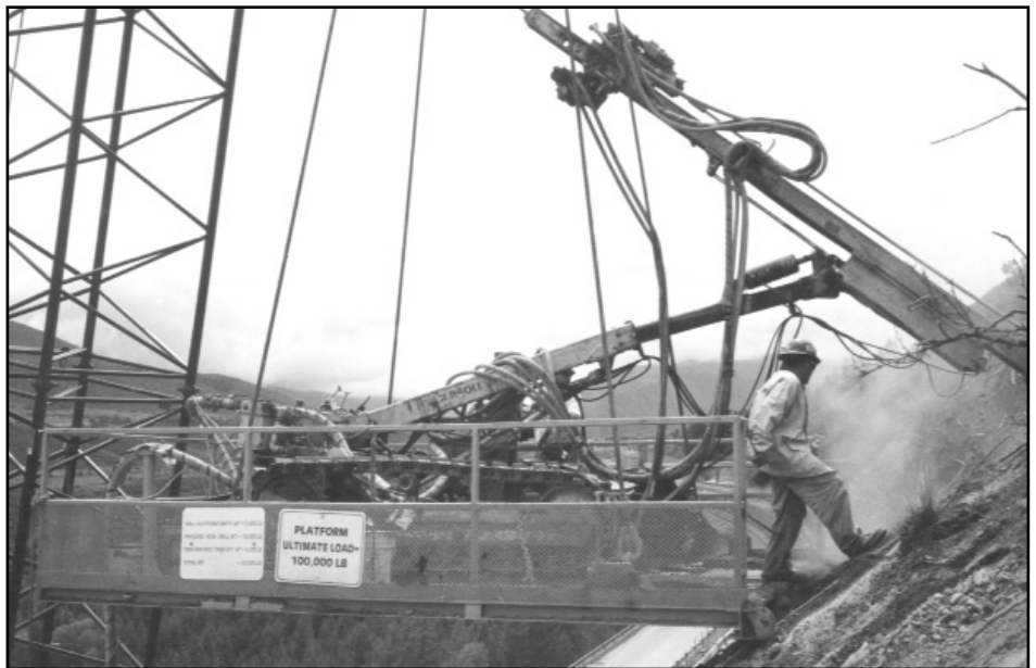
Rock anchor installation to support Mancos shale at CDOT Highway 82 Shale Bluffs project PHOTO BY R. PIHL
