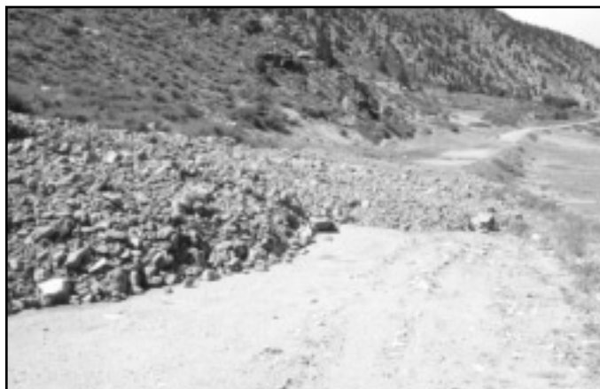
Smaller debris flows frequently cause loss of service on Colorado roads. Two examples this past summer were multiple events on I-70 near Dotsero and several debris flows on the frontage road west of Interstate 70 at Georgetown (shown above). PHOTO BY JIM SOULE
