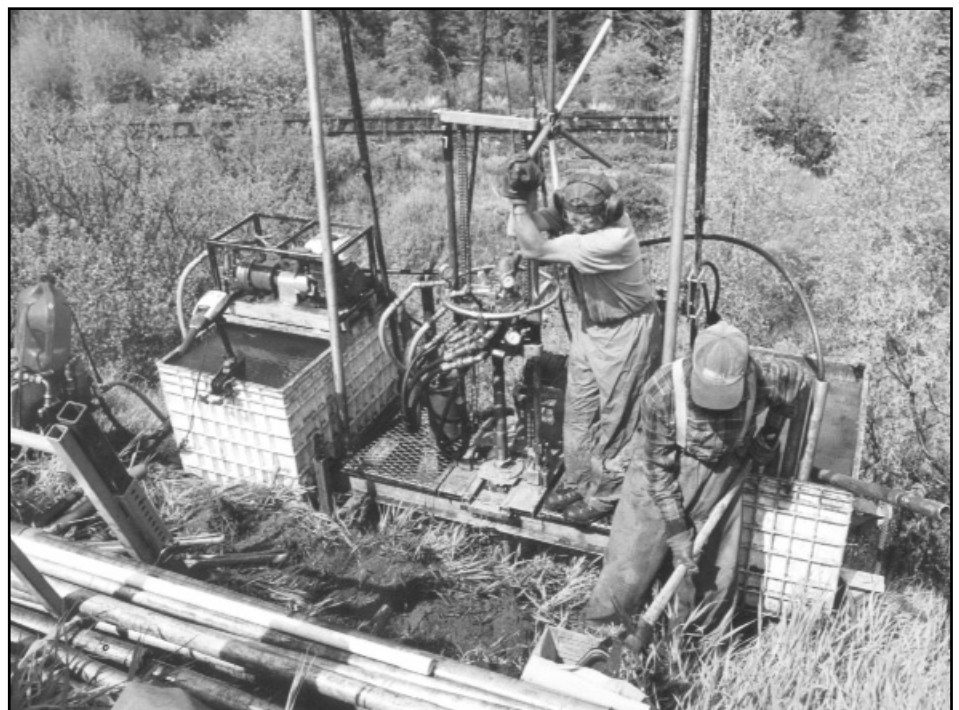
Helicopter delivered modular drills are used for access for exploratory drilling in difficult and sensitive areas PHOTO BY TY ORTIZ
