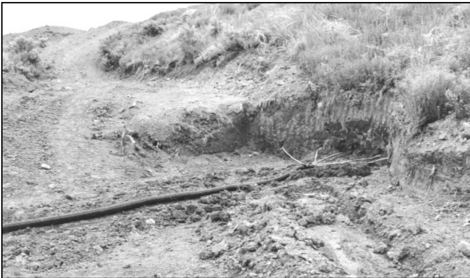
Cluster of wick drains and outfall at a State Highway 13 location PHOTO BY TY ORTIZ
