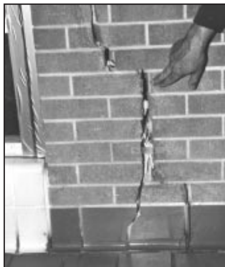
Cracks in brickwork caused by swelling soils
