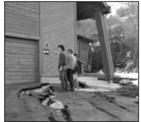
House condemned because of landslide damage
