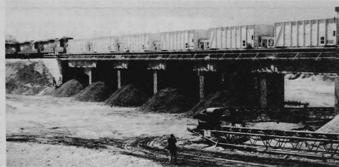
Figure 5. a) Top, Western Paving Construction Company's gravel loading facility on St. Vrain Creek at Lyons. Gravel is conveyed to a height of 65 ft and selectively dumped into the six 530-ton-capacity concrete-stave silos. Underneath, the rail cars are loaded at a rate of 200 ton/min/silo. b) Bottom, the 32 Ortner 100-ton-capacity cars are positioned on the 270-ft-long trestle to discharge the pit run into six 1500-ton-capacity bays. From there the material can be either surged to a stockpile or fed directly to the crushing and screening plant.
