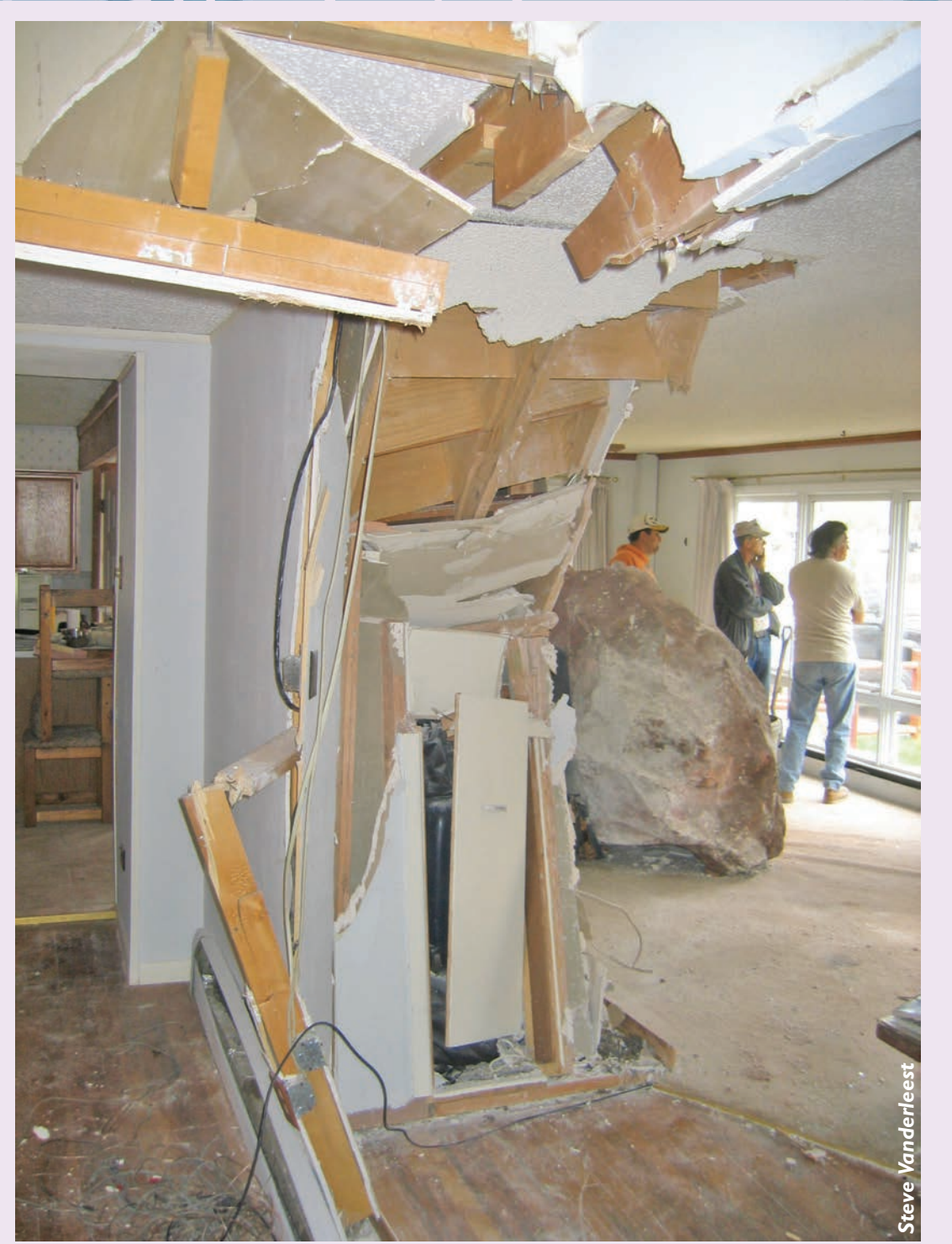
Rockfall can be a serious problem, this one occurred outside Glenwood Springs
