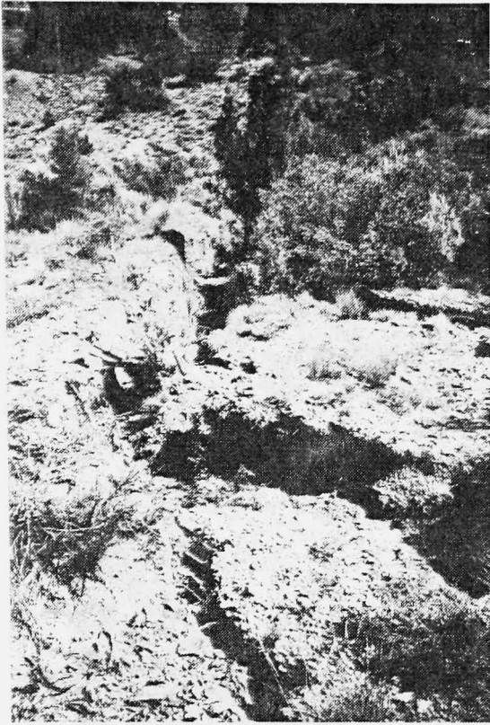
Figure 20. Tension cracks east of the slide mass. Refer to Figure 18 for location.
