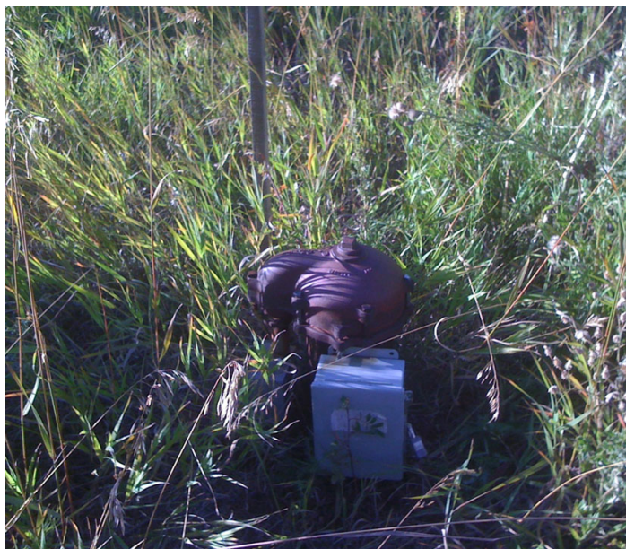
A wellhead rises about 1 foot above the ground and is capped with a sanitary seal. There also may be a conduit for wiring. Much more lies below the surface within a borehole that could extend hundreds of feet into bedrock. That borehole holds protective casing, a pump with wiring, and piping to bring water from the pump to the house.
