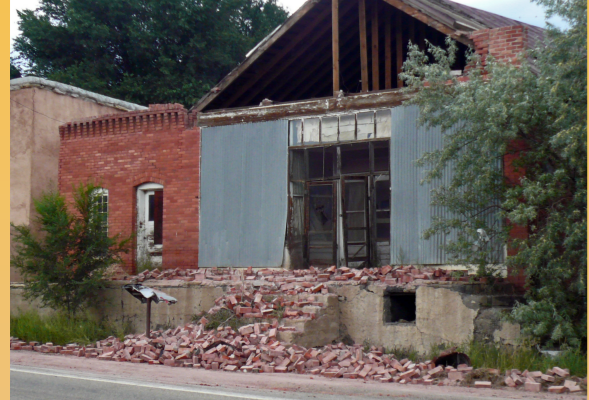
Building damaged by a magnitude 5.3 earthquake west of Trinidad, Colorado on August 22, 2011.
