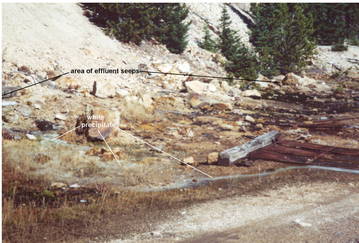
Figure 11. Effluent seeps from the caved 7D adit.
