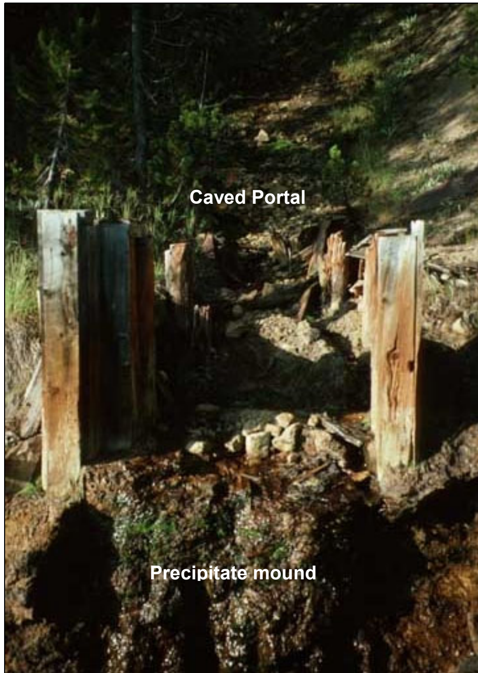
Figure 8. Photograph of caved adit #100 and precipitate mound in 1996.
