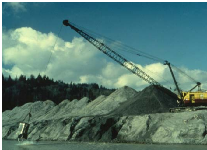
Dragline dredges St. Helens' volcanic mud from channel of North Fork of the Toutle River in an attempt to restore a navigable channel and prevent downstream sedimentation. (photo by Lynn Topinka, Cascades Volcano Observatory)
