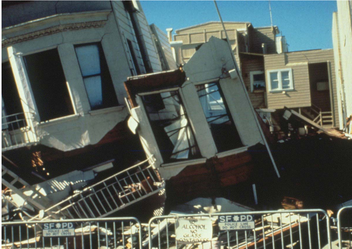
Collapsed building in the Marina District of San Francisco during the 1989 Loma Prieta Earthquake. This area was filled with sand and waste materials from the 1906 earthquake. Such fill liquefies and flows under vibration; structures such as these should never have been built on such material in earthquake country. Nine people died in fires and building collapse in this district. As in 1906, fires could not be fought with city water because shifting, liquefying ground shattered water mains. (photo from NOAA by D. Perkins, USGS)
