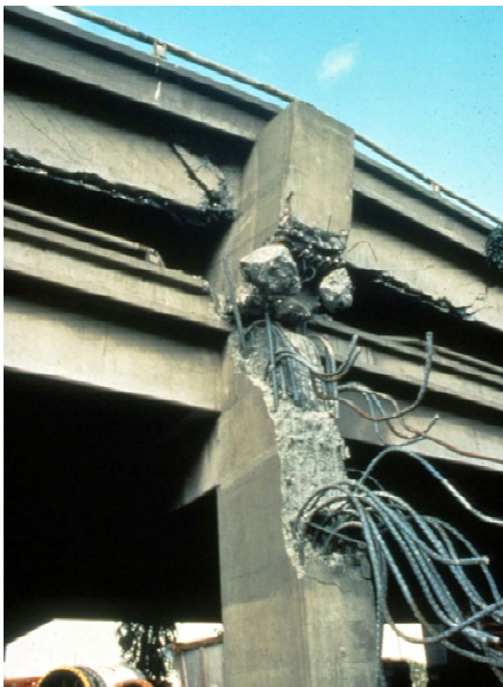
An example of tragedy from design, the upper deck of the Nimitz Freeway Interstate 880 overpass in Oakland, California, collapsed during the 1989 Loma Prieta earthquake. Column supports failed during shaking, and reinforcing bars popped from the concrete posts and peeled away like spaghetti. Elsewhere, support columns wrapped in iron withstood the vibration. These columns were due to be wrapped, but over 40 lives were lost in this collapse before action could be taken. The affected area fared well for a quake of this size, primarily due to good earthquake design practice. (photo by H. G. Wilshire, USGS)
