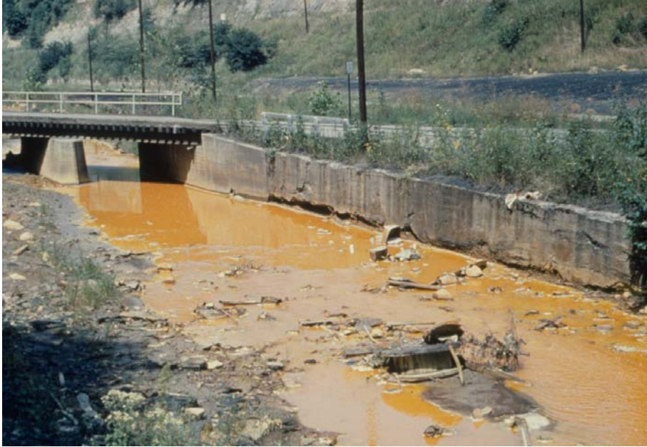
Acid drainage from old Appalachian coal mines produced the rust-red sludges in the stream. The acid water corroded the Portland cement - based concrete retainer wall, and bridge supports shown will soon share the same fate. Reclamation and mining practices now minimize acid drainage. Sites like this are rarely caused by modern surface mines. Federal and state abandoned mine lands programs are having a gradual but telling effect on restoring water quality to such streams. (photo circa 1960s from WV Geol. and Economic Survey)
