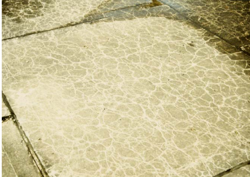
Map-cracking in this concrete reveals an expansive reaction between the aggregate and the cement within the concrete. Soon the finished surface will spall away and complete deterioration will follow. (photo by Edward Nuhfer)
