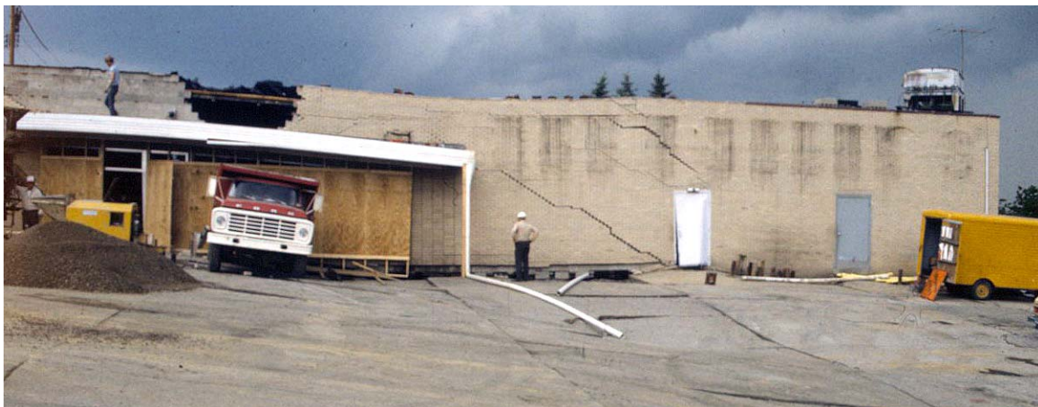
Grocery store in residential area south of Pittsburgh, Pennsylvania, subsides into an abandoned coal mine. (photo by Edward Nuhfer)
