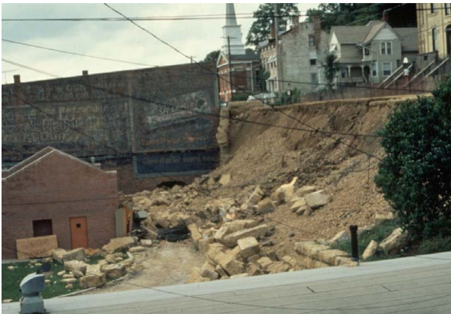
Failure to appreciate the angle of repose of fill may have led to the collapse of this rock wall in northern Illinois. Soil fill was surrounded by a stone block decorative wall of insufficient strength to act as a retainer wall. Pressure accumulated as the fill settled until it suddenly broke the wall and cast blocks and fill material onto users of the parking area below. Fatalities resulted. (photo by Richard Wetzel)
