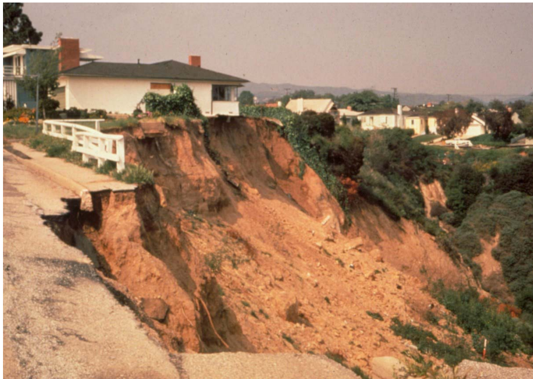
This landslide has undercut the foundation of this California home, has removed the sidewalk and threatens the road in the foreground. Landslides affect both buildings and transportation routes. Special engineering design, zoning and land use management can greatly reduce scenes such as this one. (photo by J. T. McGill, USGS)
