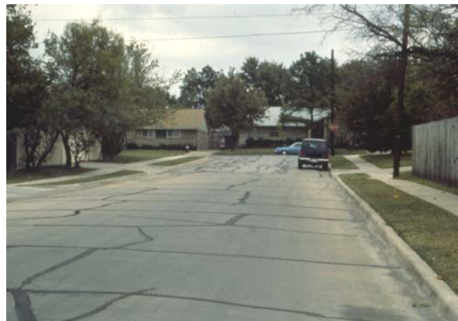
Paved roads constructed without precautions on swelling soils exhibit heaving, undulation and extensive cracking. (photo by Edward Nuhfer)
