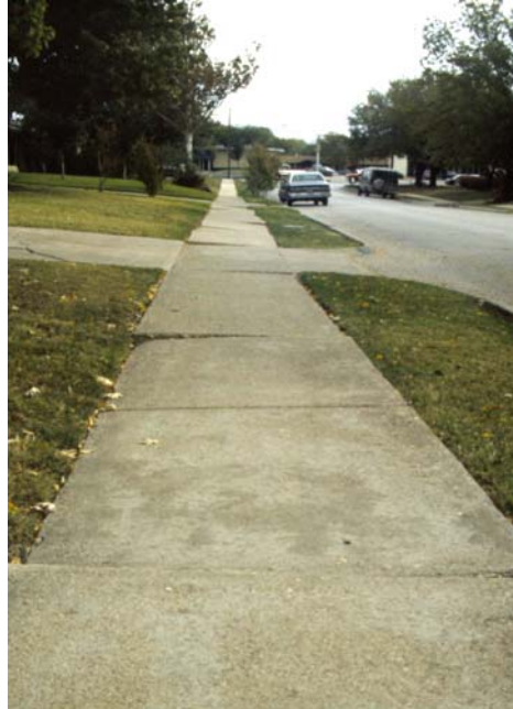
Undulation and heaving slabs distinguish this sidewalk near Dallas, Texas, as built upon swelling soils. (photo by Edward Nuhfer)
