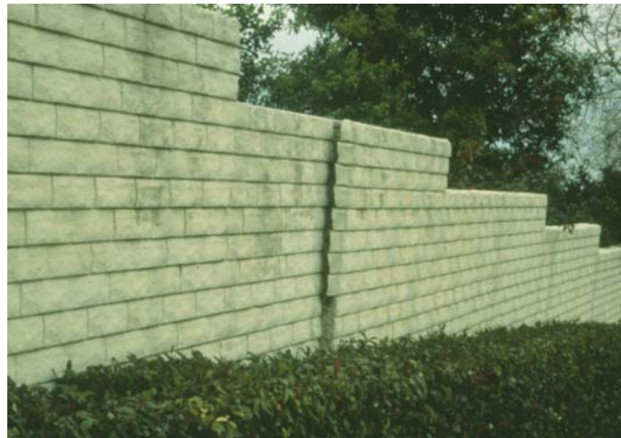
Stresses exerted by swelling soils have caused this block wall surrounding a condominium complex to tilt and break. (photo by Edward Nuhfer)
