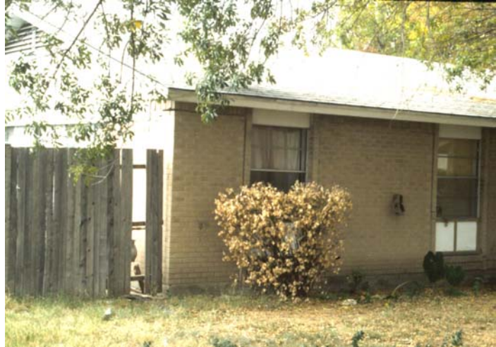
Heaving of swelling soils has damaged this Texas home, causing separation near the roof. (photo by Edward Nuhfer)
