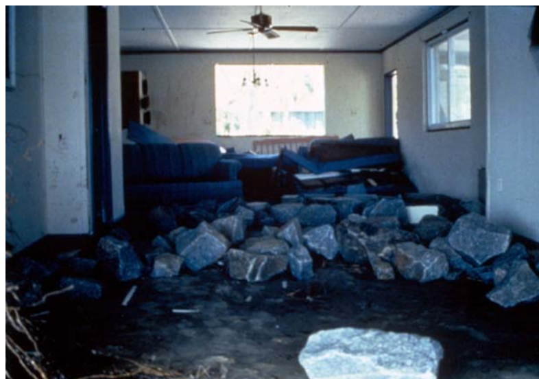
In an act with the flavor of a defiant parting gesture, Hugo deposited the riprap blocks from the barrier wall into the very living rooms of the homes the wall was intended to protect. (photos from National Weather Service, NOAA, National Hurricane Center)
