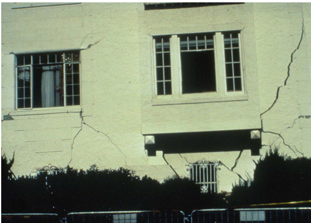
Fractures in this structure were produced by subsidence when unconsolidated sediments beneath the Pacific Garden Mall in Santa Cruz, California, settled during the 1989 Loma Prieta earthquake. (photo by C. Stover, USGS)
