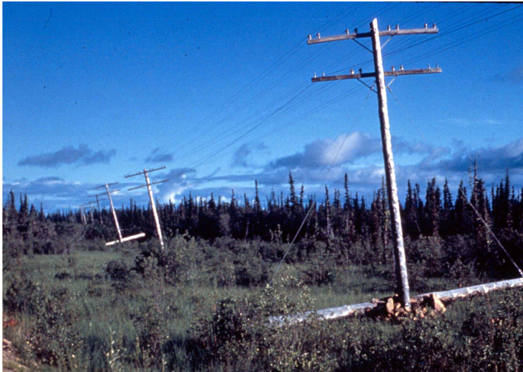
Extreme shifting and tilting of these power lines occur because of shifting of the permafrost soils in which they are set. (photo by T. L. Pewe, USGS)
