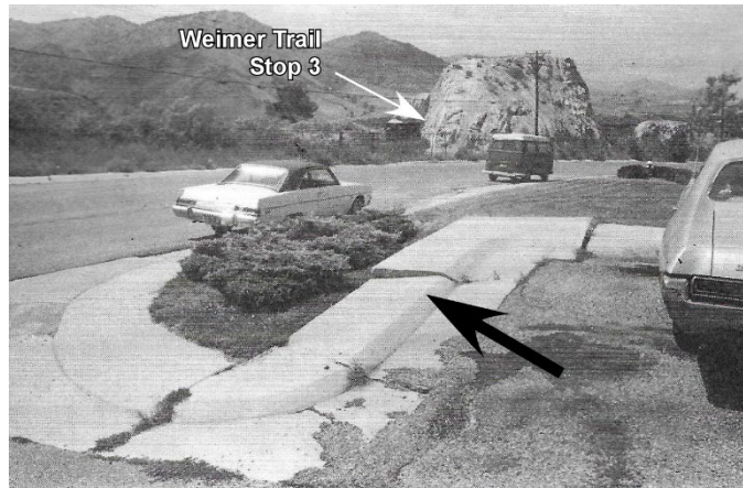
Fig. 102. Cracked and slumped sidewalk (black arrow) on the CSM campus circa 1977, caused by differential subsidence. Today's Stop 3 on the Weimer Geology Trail (white arrow) in background. Photo from Amuedo et al. (1978, p. VI-6a). View to north.
