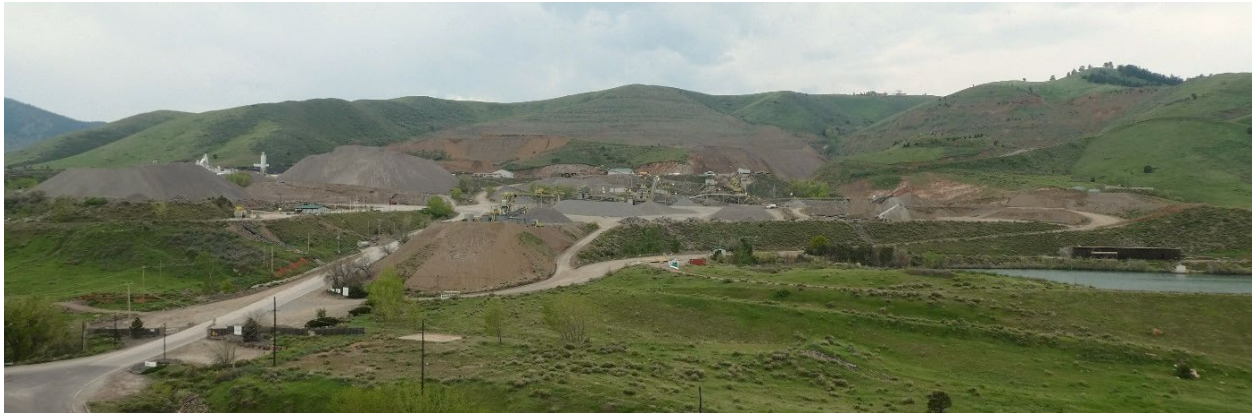
Fig. 89. The Specification Aggregate (Spec-Agg) Quarry in 2019. View to west from the south Dakota (Tincup) Hogback.
