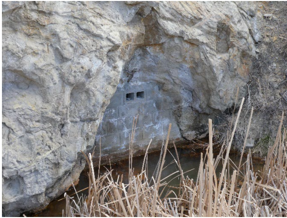
Fig. 57. Abandoned Welch Ditch tunnel portal on east side of U.S. Highway 6. Location shown in Fig. 56.
