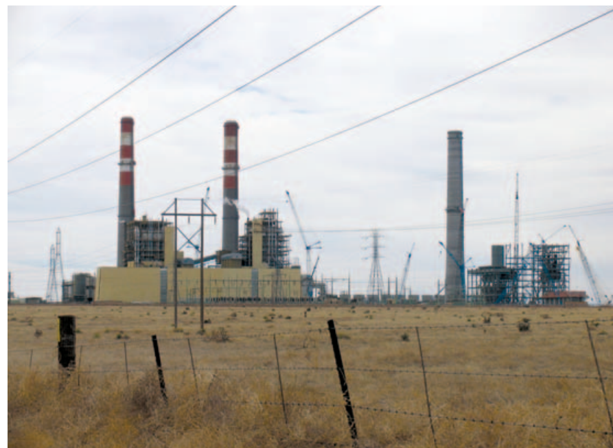
Figure 34. Construction at the new generating facility at Xcel Energy's Comanche Power Station in Pueblo County, March 2007. The new stack is located on the right.
