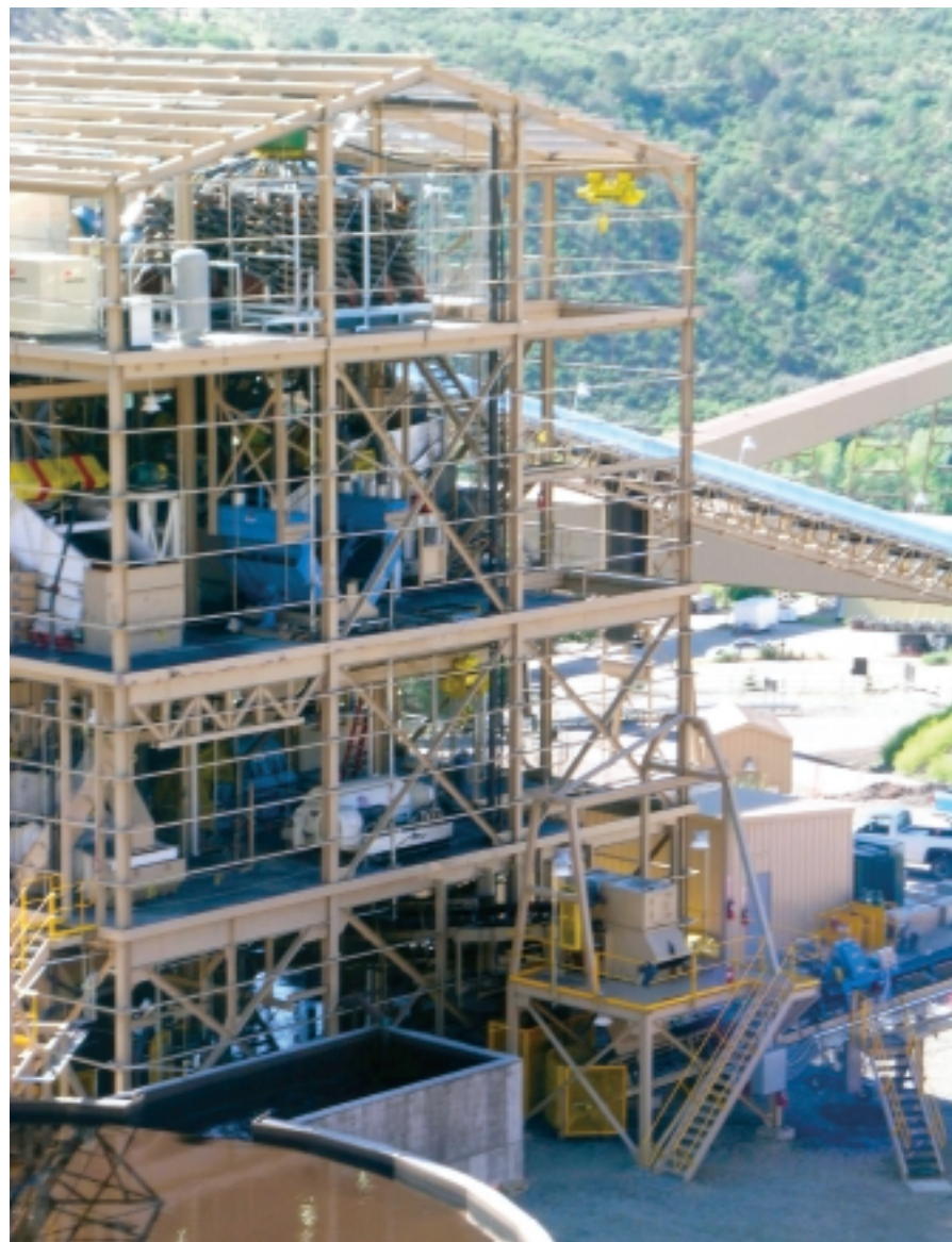
Figure 36. Construction of the new preparation plant (before walls) for the Bowie Resources Mines near Paonia, Colorado, August 2004.
