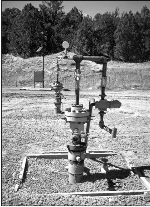
Figure 12. Coalbed methane well surface equipment (i.e., Christmas tree), La Plata County, Colorado. (Photo by Laura Wray)
