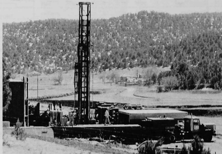
Figure 24. Pense Brothers Drilling rig setting surface casing on the Evergreen Resources, Inc. #33-32 Eureka; NE 1 / 4 SE 1 / 4 of sec. 32, T. 32 S., R. 65 W., Las Animas County, Colorado. The Eureka is planned as a 1,332 foot development well in the rapidly growing Spanish Peak coalbed methane field being developed by Evergreen Resources, Inc. in the central Raton Basin area.
