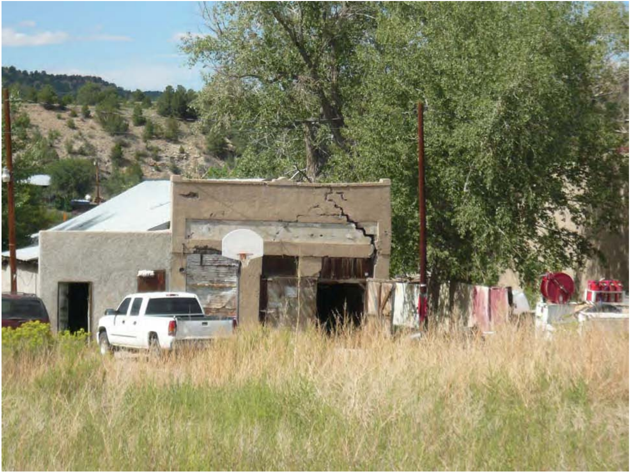
Figure 18. A severely damaged garage in Valdez, CO.
