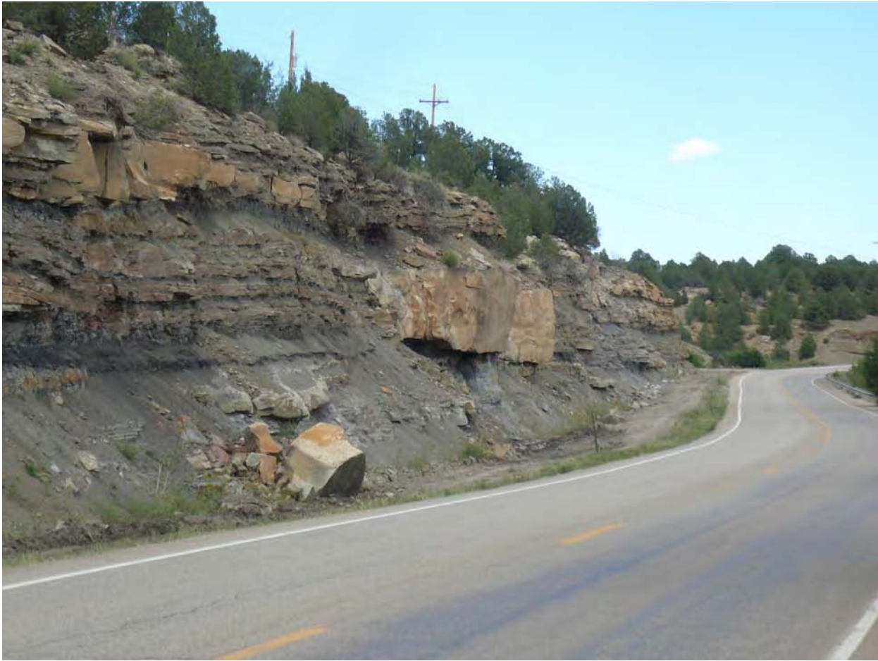
Figure 11. Rockfall events along Highway 12, east of Valdez, temporarily closed the highway. Some boulders were in excess of 6 feet across. CDOT quickly cleaned up the roadway.
