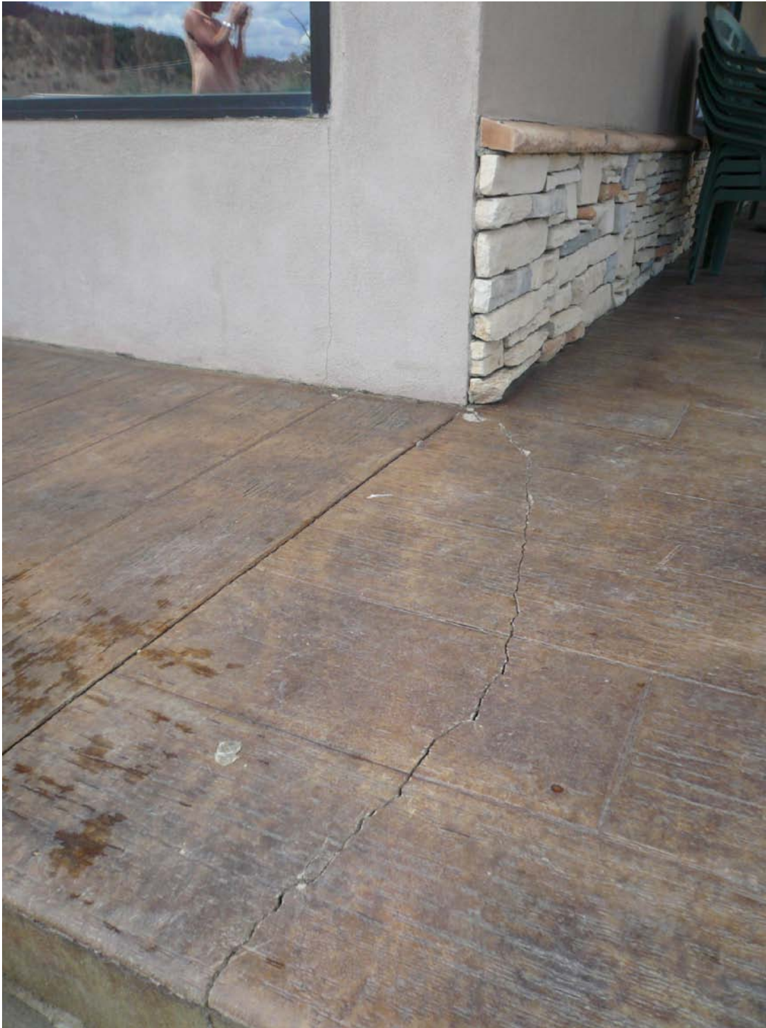
Figure 16. A five-foot-long crack in the concrete at the Big 4 Country Store in Valdez, CO.
