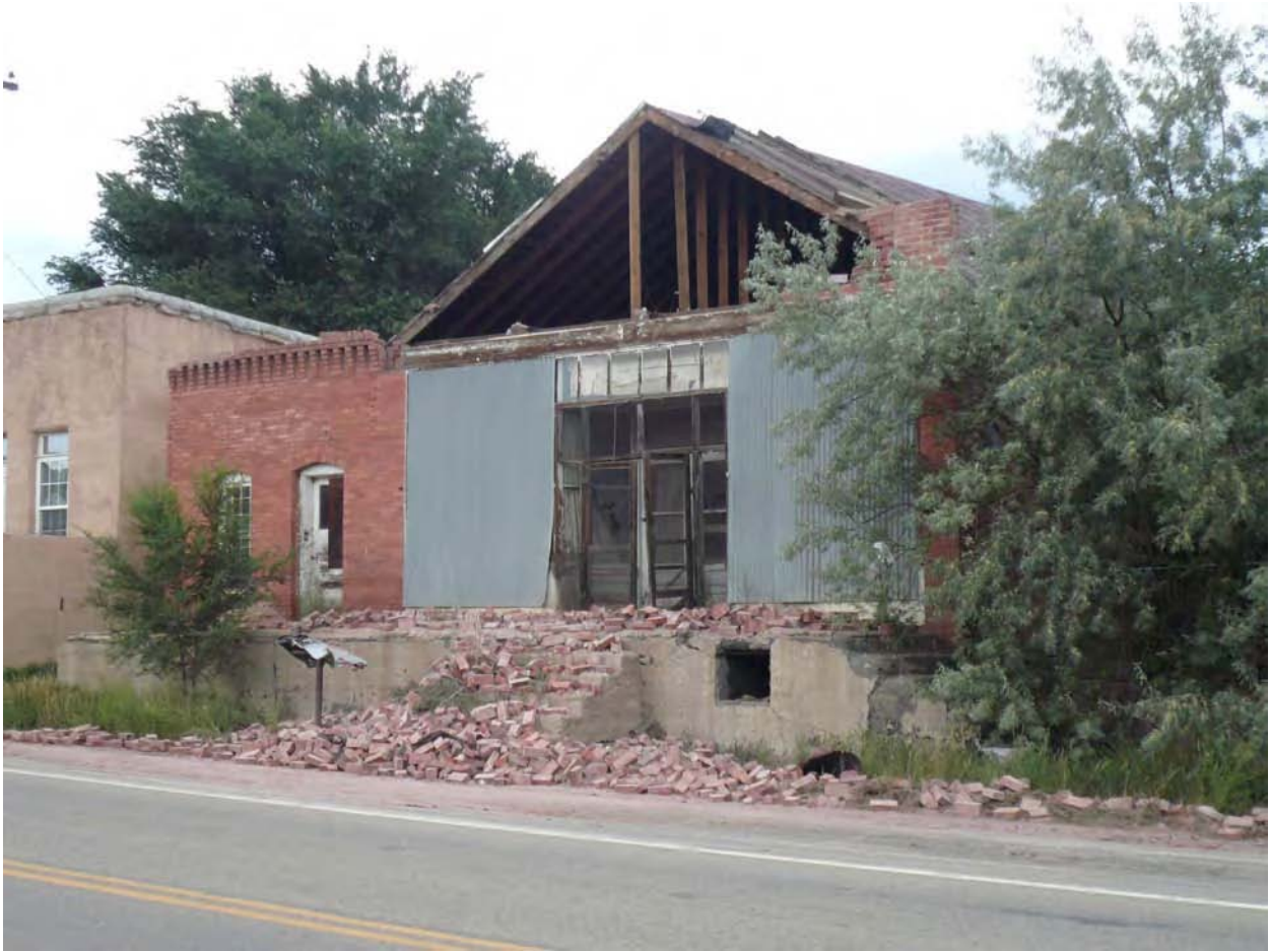
Figure 8. The front of this brick building collapsed, sending debris onto State Highway 12. Note the crushed mailbox. Segundo, CO.
