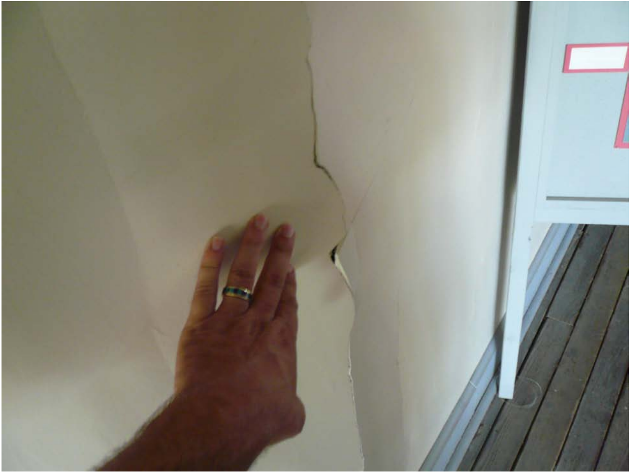
Figure 20. A few inches of buckling along the same crack in Figure 19. Cokedale, CO.
