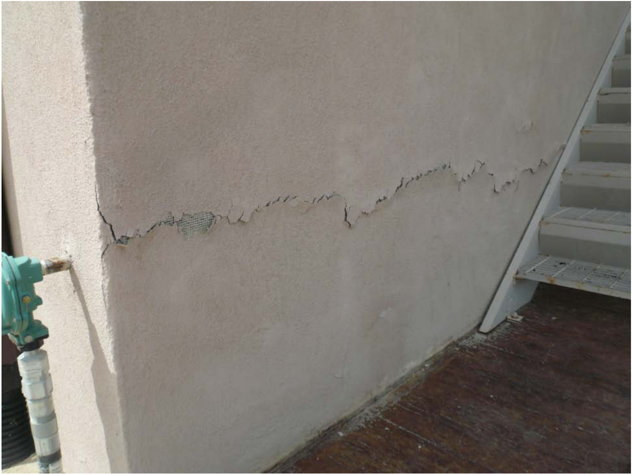
Figure 17. Cracked plaster at the Big 4 Country Store in Valdez, CO.
