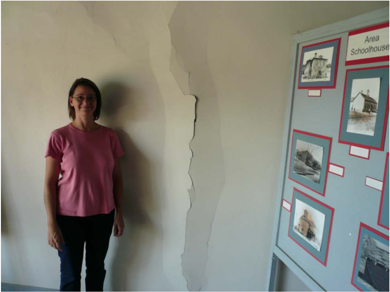
Figure 19. A 10 foot long vertical crack in the upstairs floor of the Cokedale post office/city hall.
