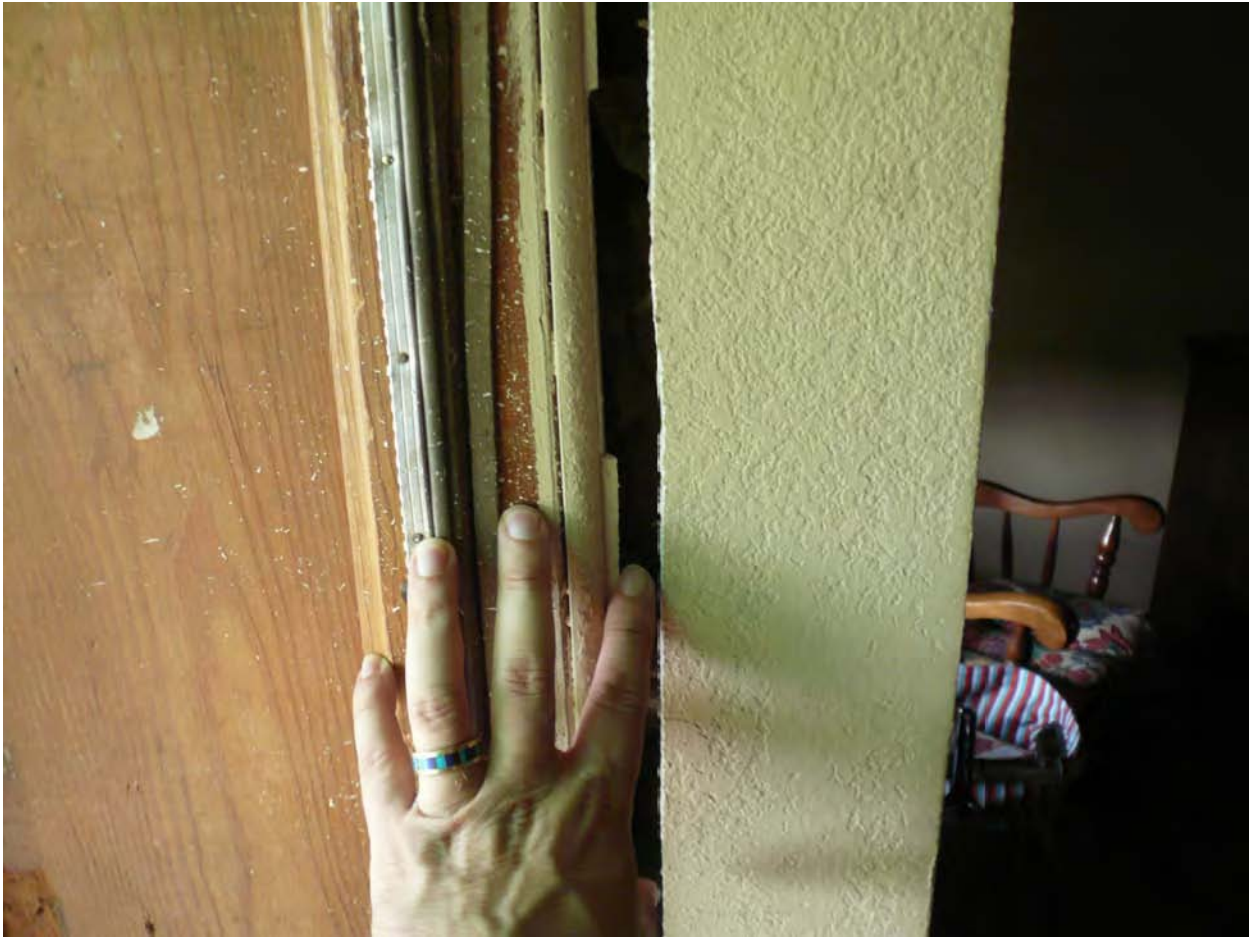
Figure 3. The exterior wall pulled away approximately 1" from the interior wall. Segundo, CO.
