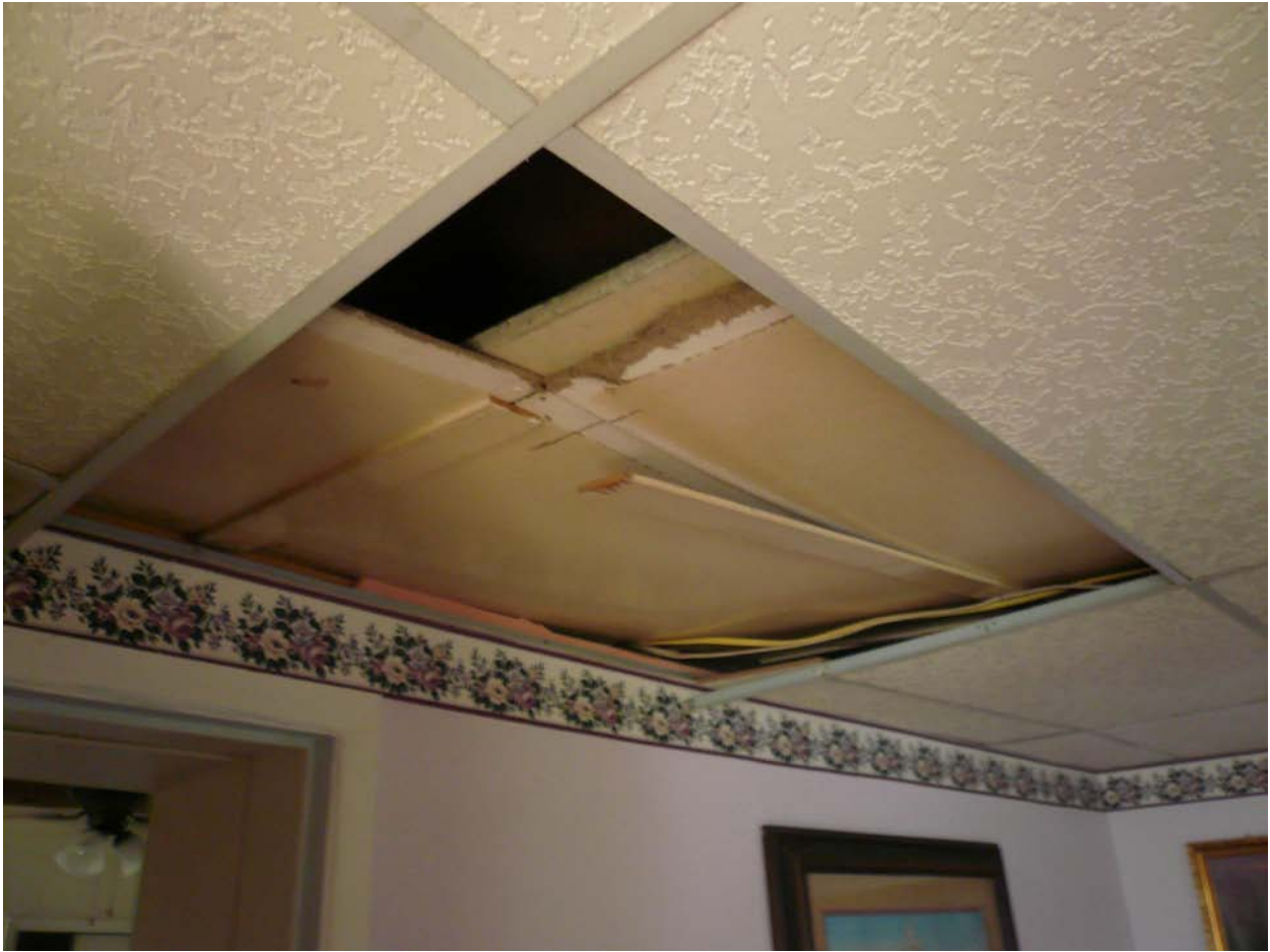
Figure 15. A ceiling panel collapsed sending debris on the resident's bed. Segundo, CO.
