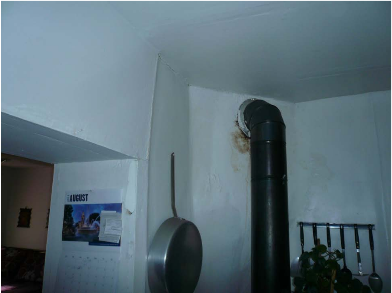
Figure 14. Chimney from a stove was pulled from the wall. Segundo, CO.
