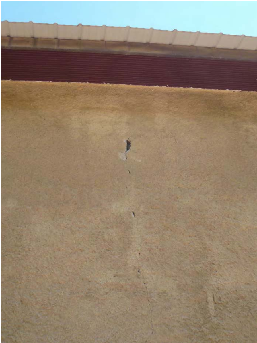
Figure 21. A large piece of plaster missing from an external crack on the Cokedale post office.
