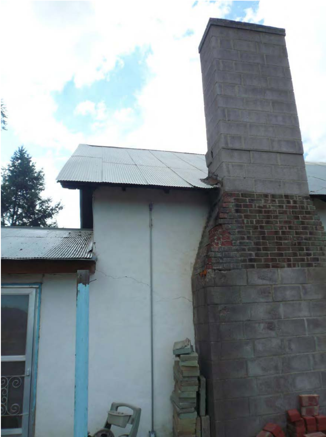
Figure 7. Chimney displaced approximately 2". Segundo, CO.
