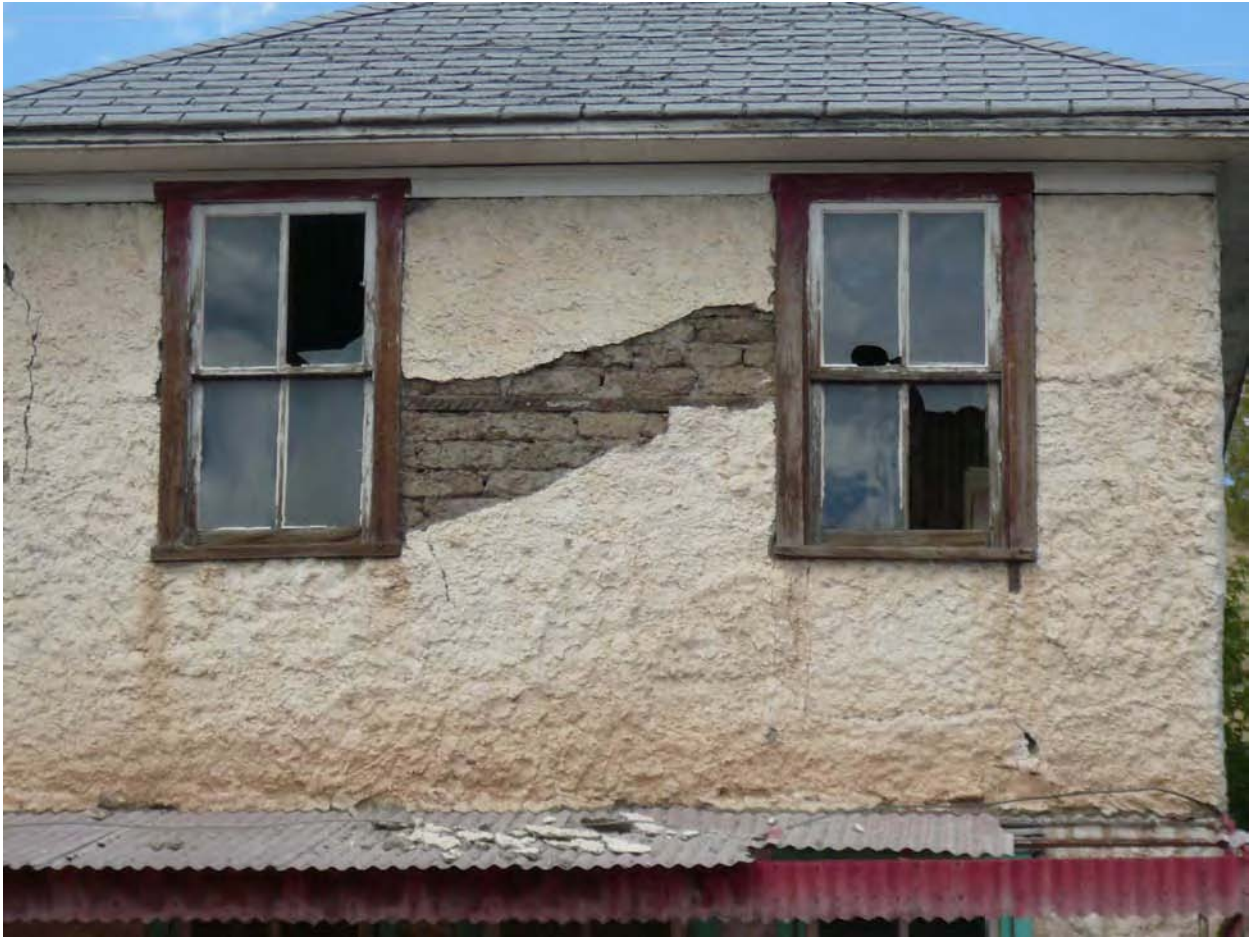
Figure 12. An old adobe building in Segundo with cracked and displaced plaster.
