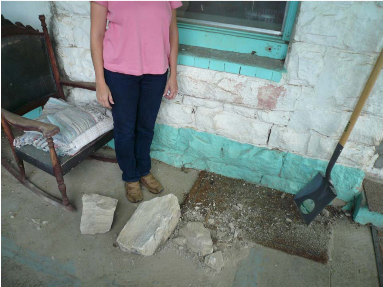
Figure 2. Two-foot-long rock blocks from the façade that fell 10 feet through the front porch roof. Segundo, CO.
