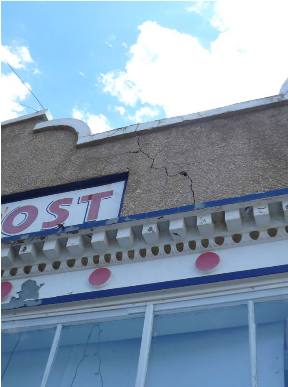
Figure 10. Cracked plaster on Ringo's Market in Segundo, CO. All of the liquor bottles inside were thrown to the floor and walls were cracked.
