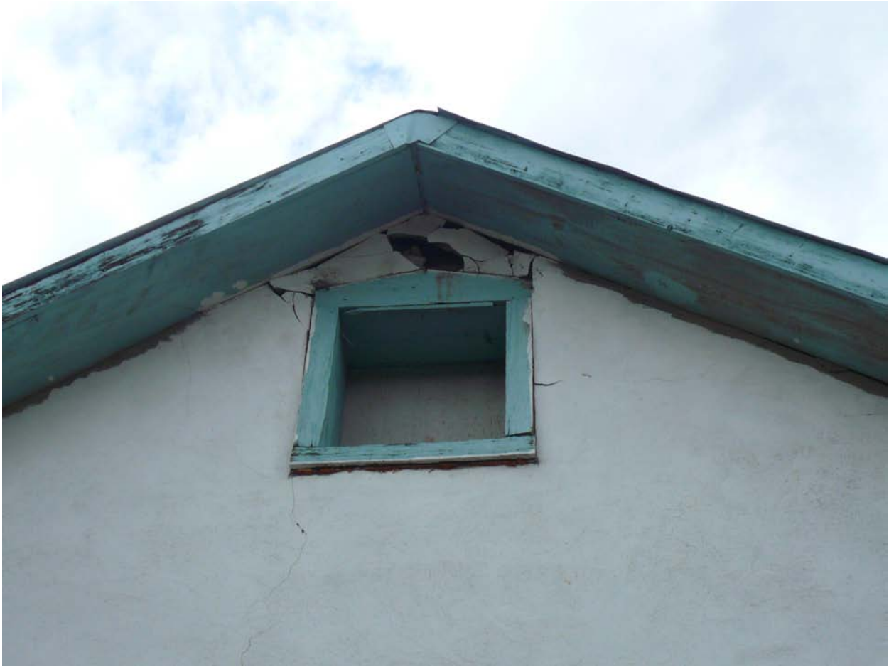
Figure 13. Major plaster and brick damage to a home in Segundo, CO.
