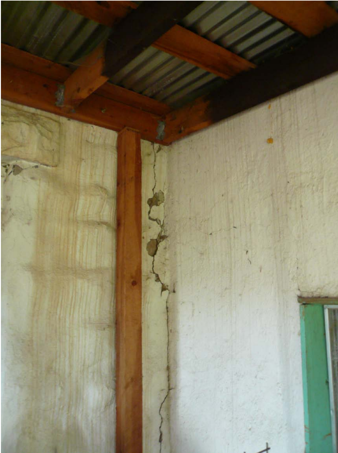
Figure 6. Cracked and missing plaster was pervasive. Segundo, CO.
