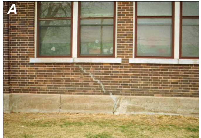
Figure 3-7. A, Typical damage to foundation walls and brickwork from settlement is visible on a school in Canon City.
