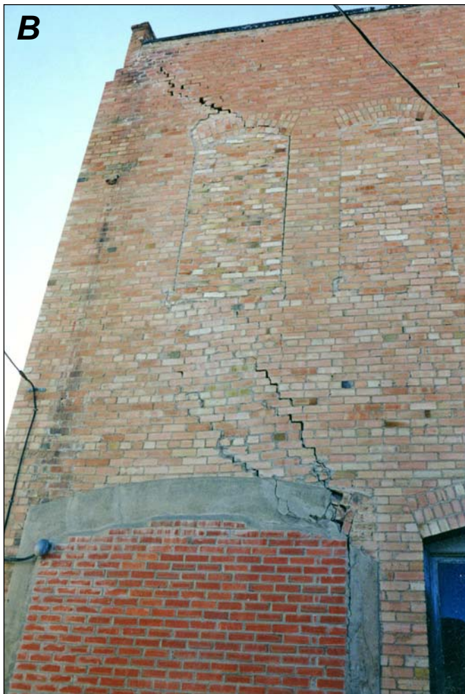
Figure 3-7. B, Extensive settlement-caused brickwork damage mars a downtown building in Montrose.
