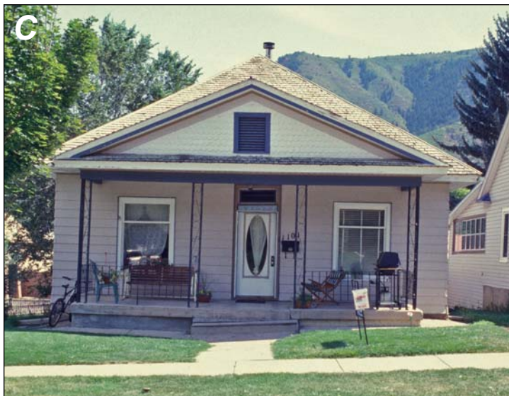
Figure 3-7. C, Settlement has damaged the porch and doorway of a home in Glenwood Springs.
