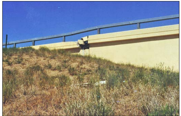
Figure 7-4. Severe settlement of bridge-abutment approach embankment, from collapse of underlying loess soil, has damaged the retaining wall and cast-in-place guardrail structure. The abutment on the right side of the photograph, founded on deep piles that were advanced through the collapsible soil, is stable.
