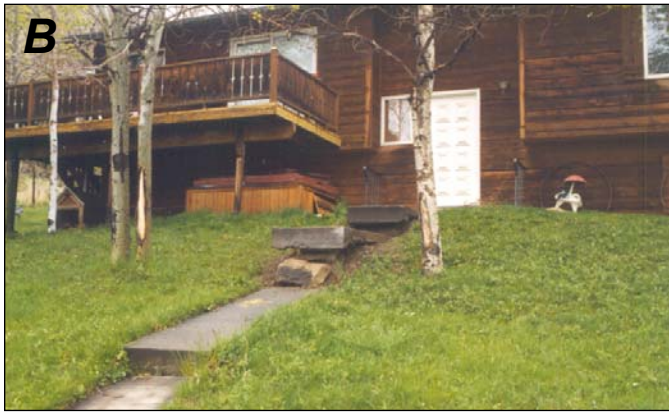
Figure 7-16. Severe settlement seen in more wide-scale subsidence in Meeker. Settlement of several feet has occurred from deep wetting of thick sections of collapse-prone alluvial-fan soils. A, Settlement and tilt of an abandoned sidewalk on the margin of a large subsidence area. Home to the right of the sidewalk (not shown in photograph) was demolished because of the extent of the damage due to differential settlement. B, Across the road on the opposite side of the subsidence area, the offset and tilt of the concrete walkway shows the extent (greater than 4 ft) of settlement of the roadway compared to the home. Note large stone used for additional step.
