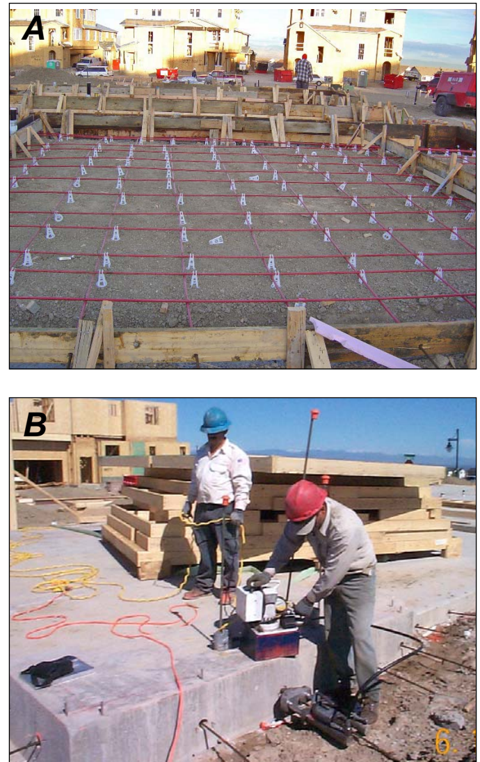
Figure 9-10. Post-tensioned slab construction. A , The prepared ground prior to concrete pour. Note the grid of high-strength tendons protected in red sheathing. White spacers act as supports and ensure proper alignment of tendons within the concrete. B , After the concrete pour, the tendons that exit the side of the concrete slab are tensioned. The worker is operating a hydraulic pump that is forcing the hydraulic cylindrical ram near the worker's foot to pull the strand. Each tendon will be tensioned and locked at a designed force or load, thereby putting the concrete into compression. Photos courtesy of Ron McOmber, CTL/Thompson, Inc.
