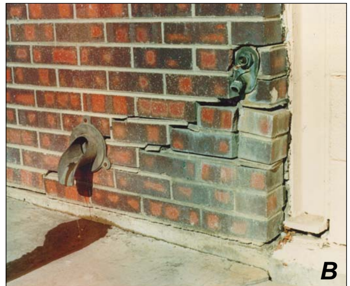
Figure 10-5. Damage to brickwork from ground settlement related to poor drainage. A , Note the gap between the brickwork and the concrete footing below at the location of the roof downspout at the Harriman School in Canon City. At the time this photograph was taken, the brickwork was still intact at this location. However, distress and signs of further foundation movement were seen in other parts of this school (fig. 3-7A). B , By comparison, this photograph shows a more severe effect of concentrated roof runoff that easily seeped to the subsoils. Note the offset of the sidewalk and foundation wall, which settled and resulted in severe distress of the brickwork. This structure at the Montrose Armory was condemned and demolished shortly after this photograph was taken. Photo courtesy of Tom Griepentrog, Buckhorn Geotech.
