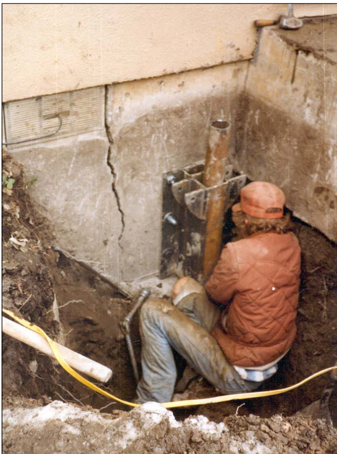
Figure 9-12. Excavation and attachment of steel bracket to a foundation wall using concrete expansion bolts. A steel pin pile is in the frame. Note settlement distress crack in the foundation wall. Photo courtesy of Steve Pawlak, HP Geotech, Inc.
