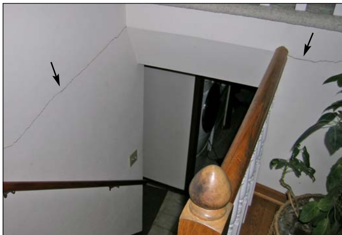
Figure 7-3. Crack in drywall (shown by arrows) formed by settling of the lower stairway wall in the foyer that is supported by a slab-on-grade foundation. The upper wall (above the crack), supported by floor joists that span to load-bearing walls at the foundation perimeter and mid-home-bearing beams, is not affected by the settlement.
