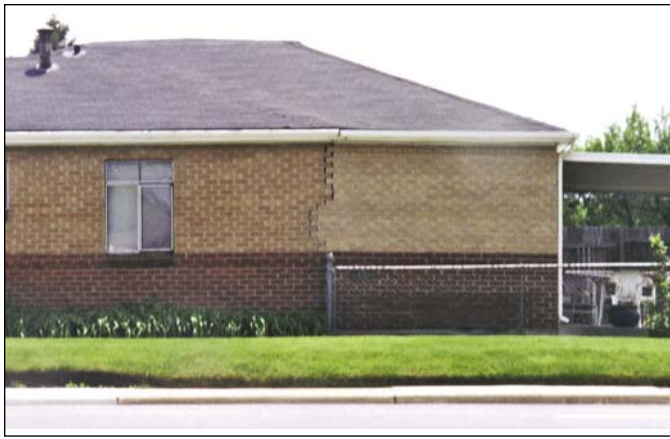
Figure 7-2. Differential settlement of the back side of this home, possibly a later addition, has unhinged house and caused distress to the brickwork and roof. The underlying soil is loess.
