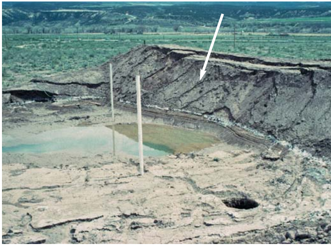
Figure 3-4. Ground settlement during a soil-flooding test near Rifle. Hydrocompaction has created arcuate, concentric ground cracks in the 10-ft-high test embankment adjacent to the pond (see arrow). Note collapse features in floor of pond due to piping erosion. Photo courtesy of R. Barrett and CDOT.
