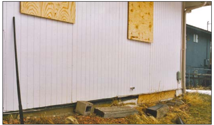
Figure 7-15. This home in Meeker was condemned and subsequently demolished because of settlement of hydrocompressive soils. Note the gap between the subsided foundation and the home's exterior wall.
