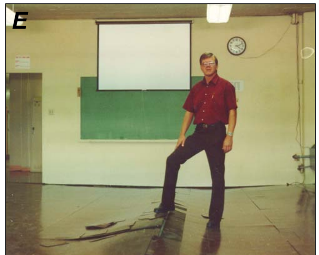
Figure 3-7. E, The wood flooring in a school in Montrose has buckled because of compression due to settlement of the underlying concrete slab-on-grade. Photo courtesy of Tom Griepentrog, Buckhorn Geotech.
