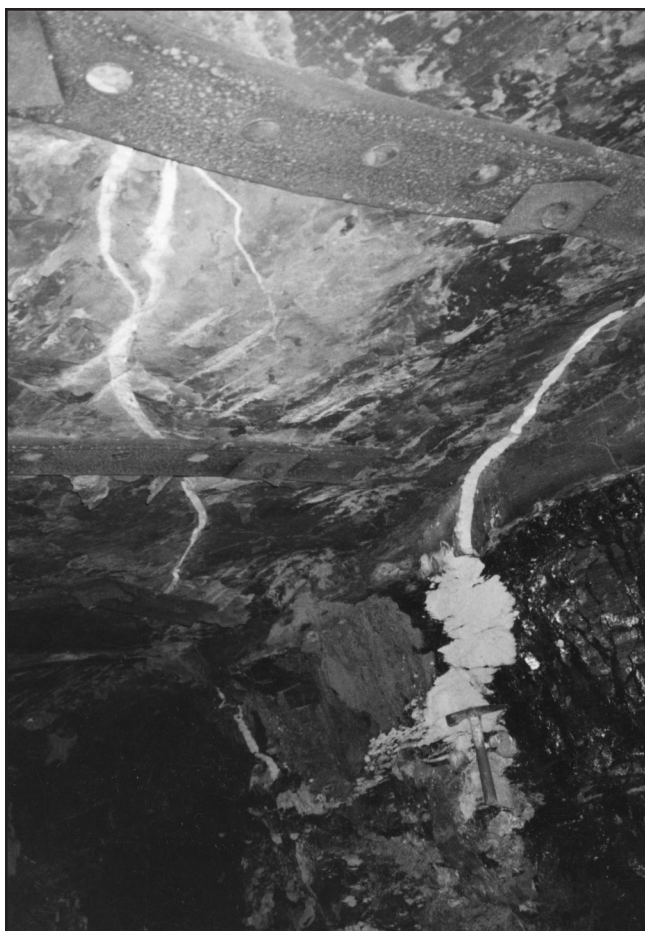
Figure 15. Photograph showing dike material that formed a splintered pattern across the roof of the Roadside (south) Mine and that resemble infilled fractures.
