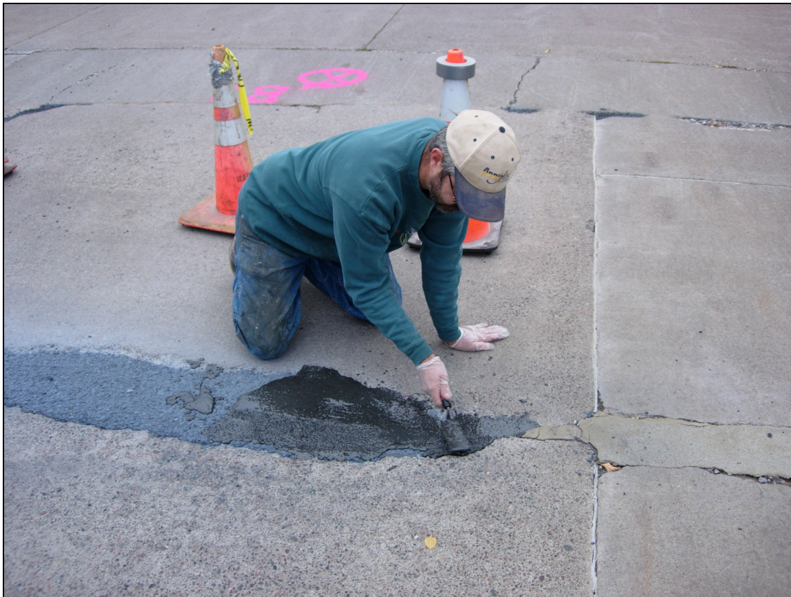
Figure 13. Top-coating of non-asphalt taconite-based patching compound at the Federal Building in Duluth, MN.
