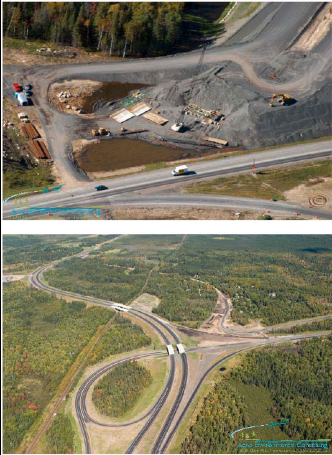
Figure 3. Coarse taconite tailings used in U.S. Hwy 53 / 169 interchange project north of Virginia, MN, 2004-2005. Upper photo shows tailings used as base material for bridge abutment construction. Lower photo is viewing north of main intersection loop (Oreskovich and Patelke, 2006). Photo used with permission: photographer David A Witt/Aero-Environmental Consulting http://www.aero-environmental.com .
