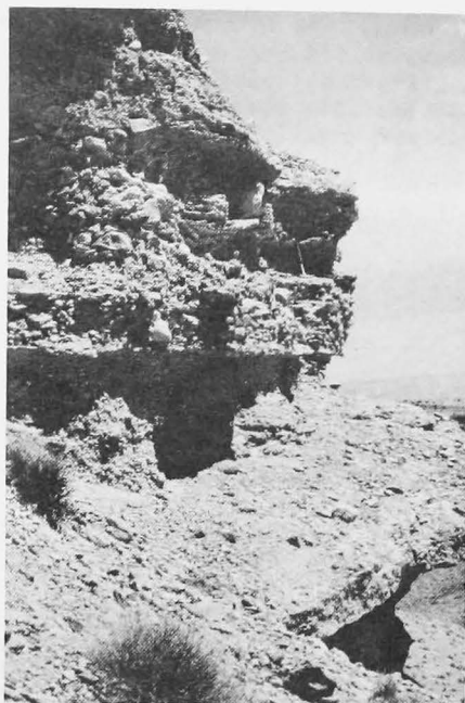
FIGURE 41. Profile of well-cemented alluvial fan gravel and conglomerate near West Salt Creek. Note the varying grain sizes from layer to layer and the different degrees of cementation and expression. Mancos Shale underlies the gravel in the lower right corner of the picture.
