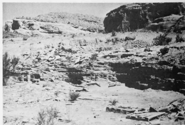
FIGURE 29a. Working face at the Loma sandstone quarry. This northwestward view is across the upper of two benches cut into the Kayenta Formation. The thin, evenly bedded, flaggy nature of the reddish-brown stone is readily apparent on the out face. The massive, light-colored Entrada Sandstone forms the prominent ledge in the left background.
