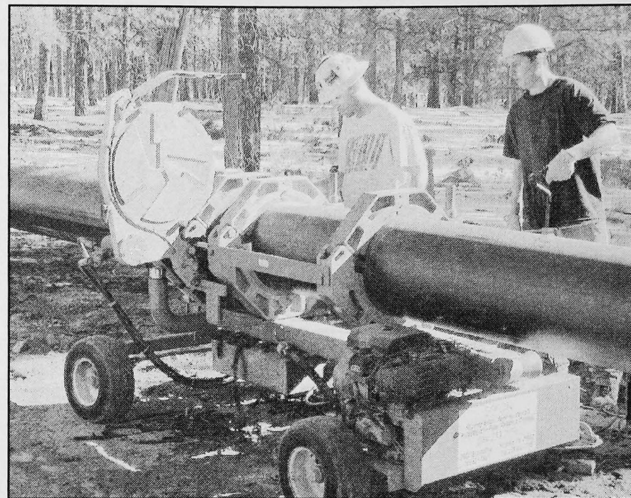
Figure 21. Fusing 16-inch poly pipe for a new, low-pressure gathering trunk line, Raton Basin, south central Colorado (photograph courtesy of Robert Mueller, Barrett Resources).
