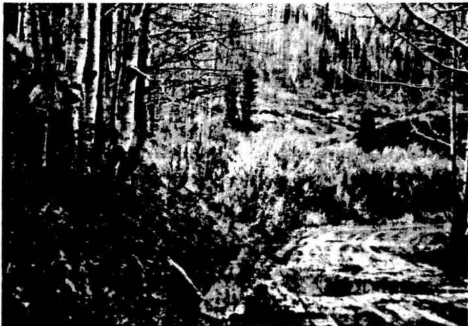
FIGURE 3. The slope to the left of the road is failing rapidly as evidenced by the curved trunks of the aspens. Note water on road that results from leakage of excess soil moisture from slope at left. (105-mm lens)
