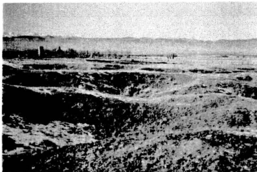
Figure 12. Large, well-developed subsidence pits over rooms of the Shanahan mine. Pits are eight to ten feet deep and are 15 to 25 feet across. The coal seam at this mine was unusually thick (10 to 15 feet), which accounts for the large amount of vertical subsidence. The mining depth was less than 50 feet. Locality 21, subsidence-inventory map.
