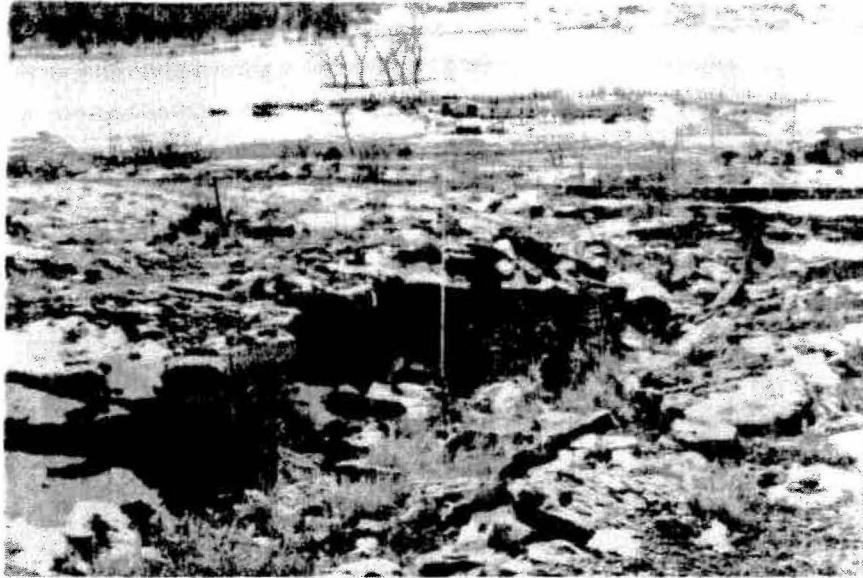
Figure 9. Collapse over room of Lewis No. 1 mine. Pit is about ten feet by 15 feet and is three feet deep. From five to ten feet of coal was extracted at a depth of approximately 50 feet. Flume carrying irrigation water in middle background must be periodically re-set because underground mine fires in this area are causing continued subsidence. Locality 7, subsidence-inventory map.
