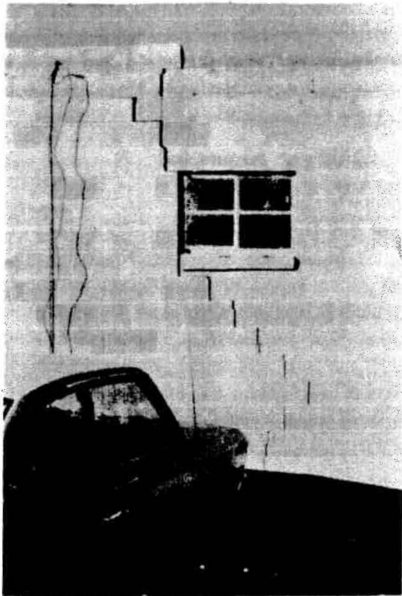
Figure 27. Damage to VFW hall, Main Street, Louisville. This part of Louisville was undermined many years ago. A seam 10 to 15 feet was extracted at a depth of about 100 feet. Because the mining occurred so long ago, it is thought that the damage to this relatively recent building is related to faulty design or construction, rather than to subsidence. Locality 43, subsidence-inventory map.
