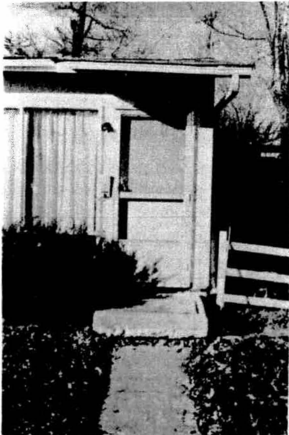
Figure 22. Front stoop of house to the right in Figure 21. This house is immediately south of home shown in Figure 20. The walk has pulled away from the stoop and it in turn has pulled away from the house. Bricks have been jammed beneath the house and beneath the stoop for temporary support. Locality 55, subsidence-inventory map.
