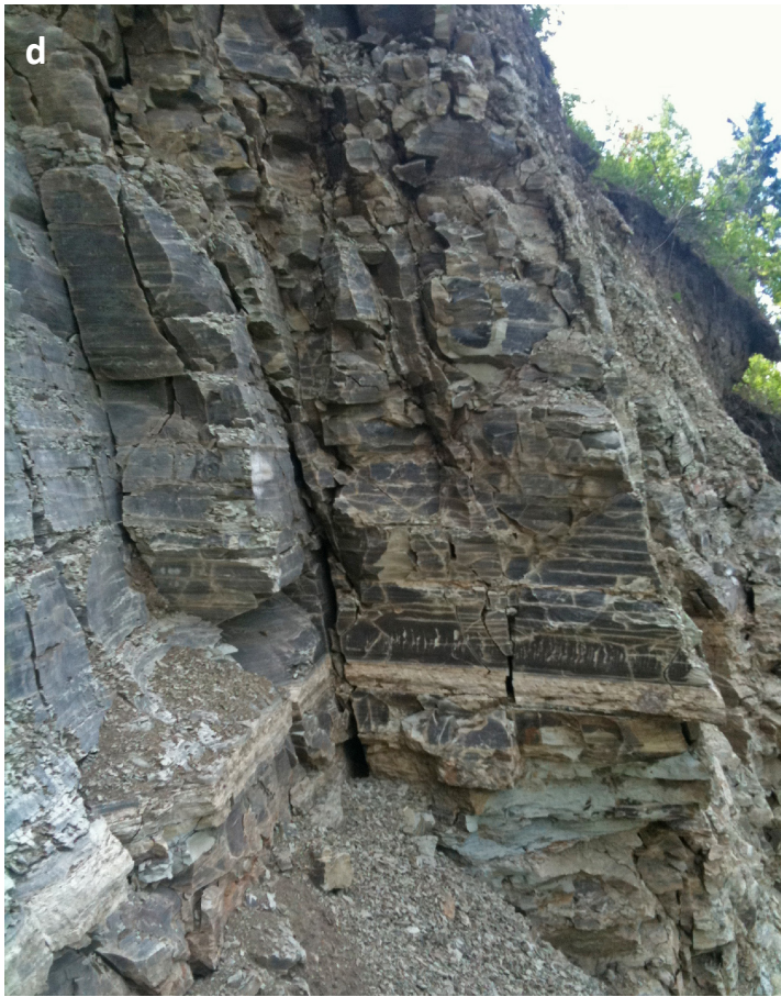
Figure 6(d). Exposed Green River Formation on west flank of scarp. Note blue-gray staining and degree of fracturing in the rockmass. Photos taken summer of 2014.
