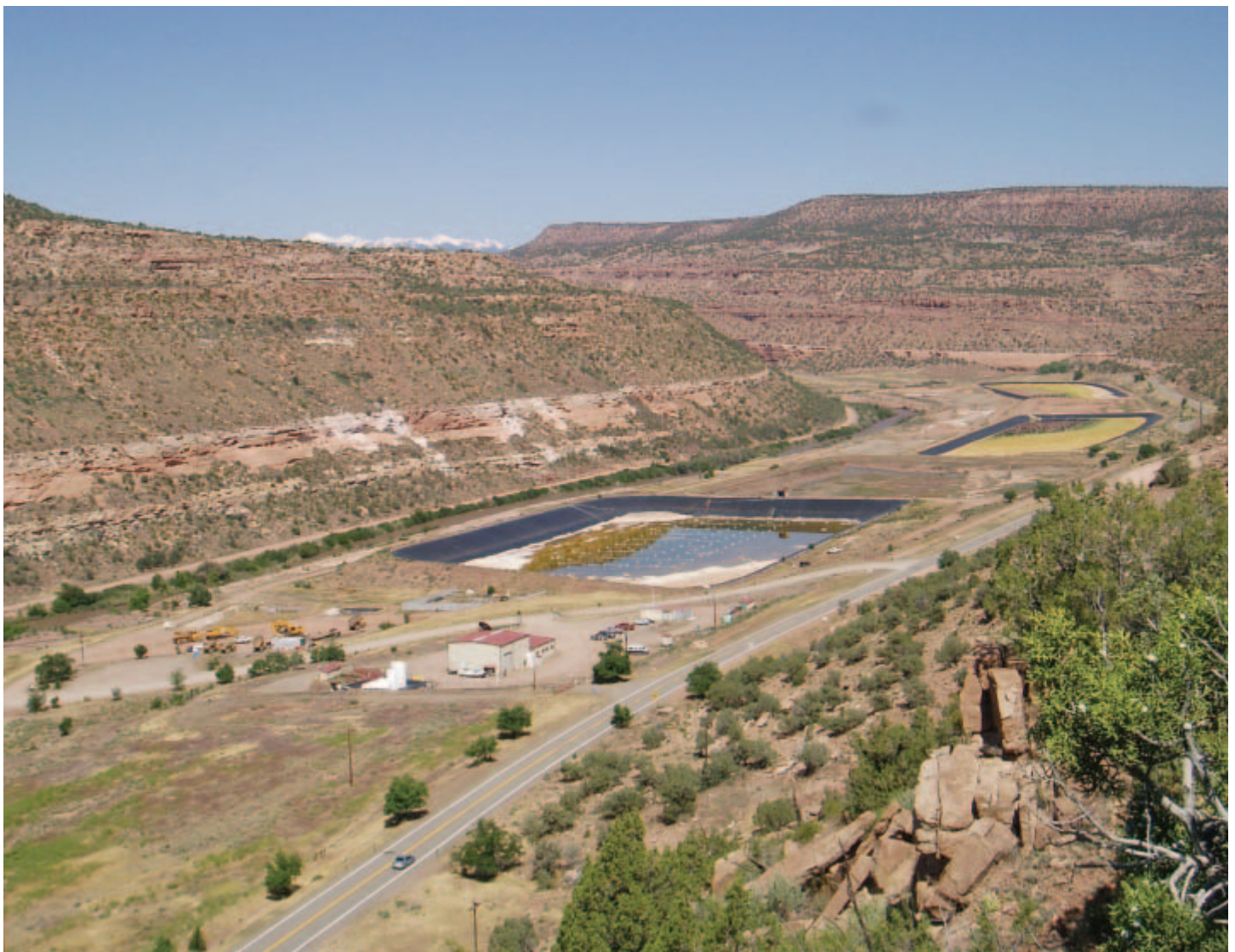
Figure 10. The Uravan site in Spring 2005; cleanup work is almost complete. Compare this photograph to Figure 7; both were taken from approximately the same point.
