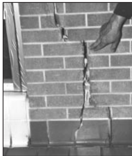
Cracks in brickwork caused by swelling soils
